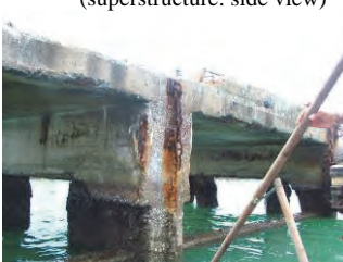
(17) Oil Jetty-6 (missing fender system)
