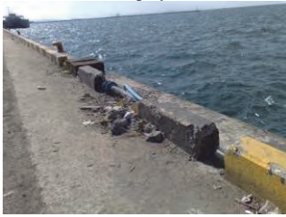
(4) New Quay-4 (broken concrete curb)
