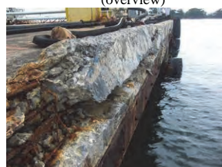
(15) Oil Jetty-4 (broken concrete curb)
