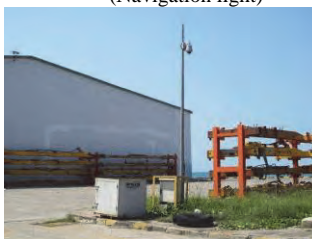
(14) CCTV System-1 (CCTV camera)
