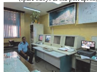
(15) CCTV System-2 (CCTV control room)
