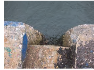
(3) New Quay-3 (missing ladder)
