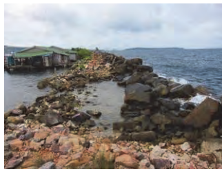
(2) North Breakwater (N)-2 (lacking stone fills portion)
