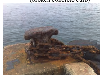
(18) Oil Jetty-7 (rusted bollard)
