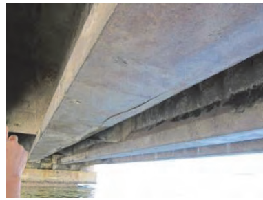
(31) Cracked P/C Beam (Access Brdg.) Type 1-3 (Epoxy, Epoxy Mortar)
