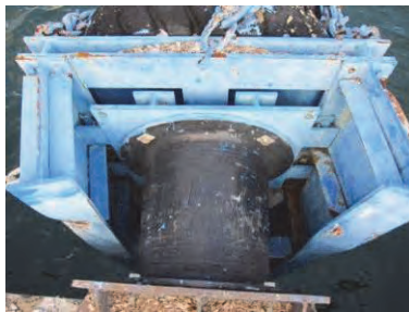
(7) Circular Fender (offshore side) Seriously damaged
