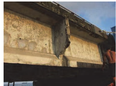
(42) Damaged Traverse P/C Cable Concrete Encasement (MP/inshore)
