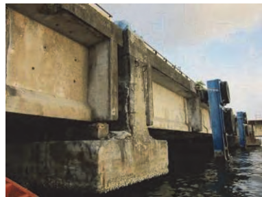
(40) Damaged Abutting Beam (MP/inshore), Rebars exposed
