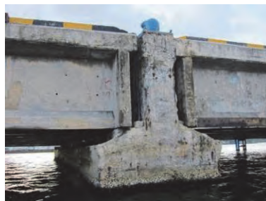
(44) Damaged Abutting Beam (MP/offshore), Rebars exposed & rust fluid
