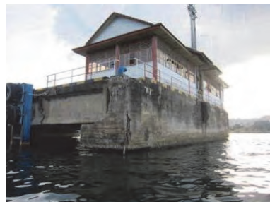
(43) Damaged Abutting Beam (MP/offshore), Rebars exposed & concrete deteriorated
