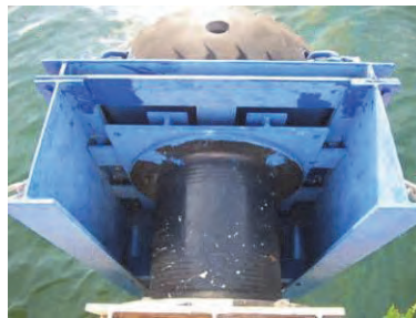
(8) Circular Fender (inshore side) Minor crack
