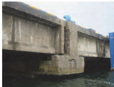
(41) Damaged Abutting Beam (MP/inshore), Rebars exposed
