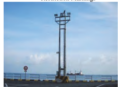
(15) Apron Lighting System CCTV camera attached
