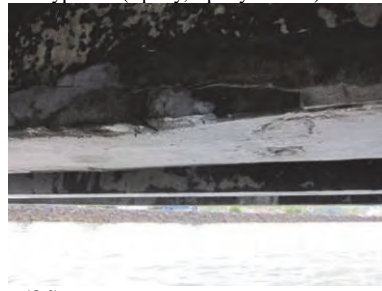
(34) Damaged P/C Beam (Access Brdg.) Type 1-2 (Epoxy Mortar)
