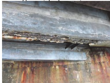
(38) Damaged P/C Beam (Cnr. Junction) Type 2 (Epoxy Mortar)
