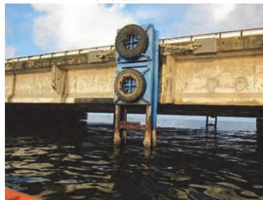
(11) Fender Supporting H-Piles (inshore side) , Rusty
