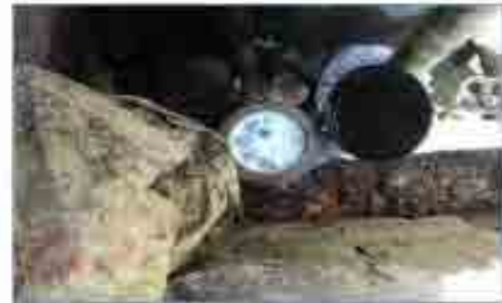
Photo of Service Meter
