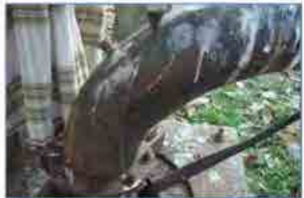
Deep Well Location (90° Bend)
