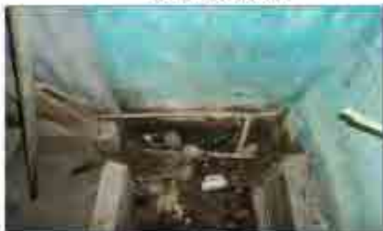
Photo of By Pass Line
