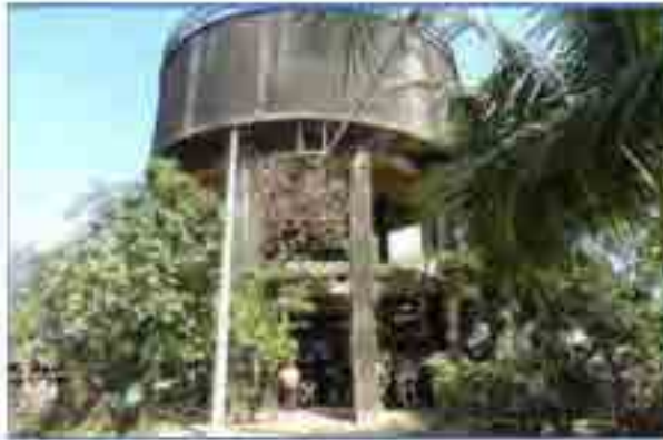
Over Head Tank Location
