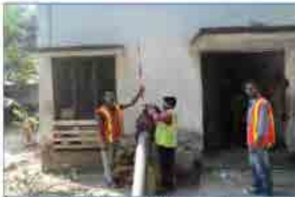
Gate Valve (Deep Well Location)
