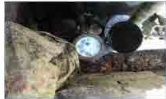
Photo of Service Meter
