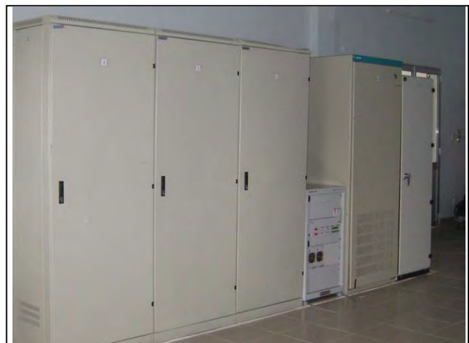
Photo 4.4-3 SCADA System installed in the Electrical Control Room in 500kV Switchyard
