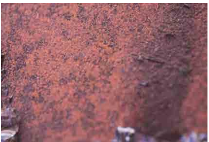
Rust generation general (※5)
