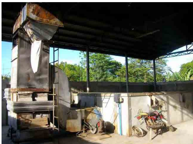
Rice dryer installed by DA for Rinconada Integrated NIS in Camarines Sur, Region-5. Drying fee is collected from users and becomes income source of Irrigators Association.
