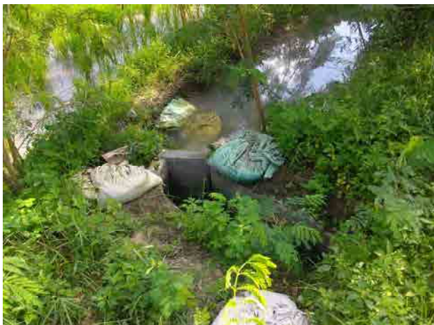
Turn-out on the lateral canal of Porac-Gumain NIS. Maintenance works are made by IA farmers to keep its function.
