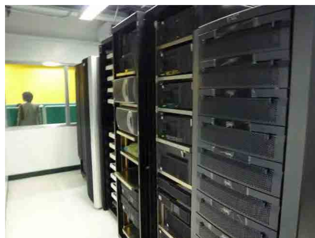
Inside Data Center of DA-ITCAF. In this server, various sources of AFMIS, data warehouse and website of Regional Offices are installed.
