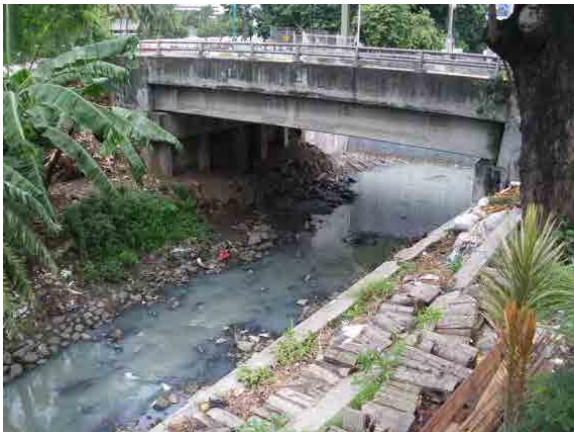
Influent channel into the existing Setiabudi WWTP.
