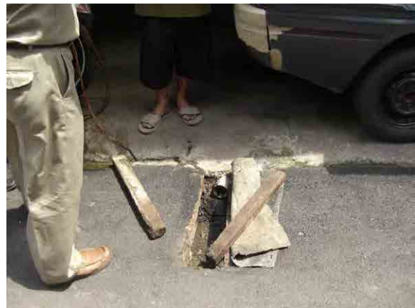
Gray water flowing into drainage from septic tank.
