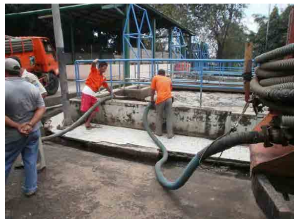
On-site sludge is discharged into receiving tank at the existing sludge treatment plant.
