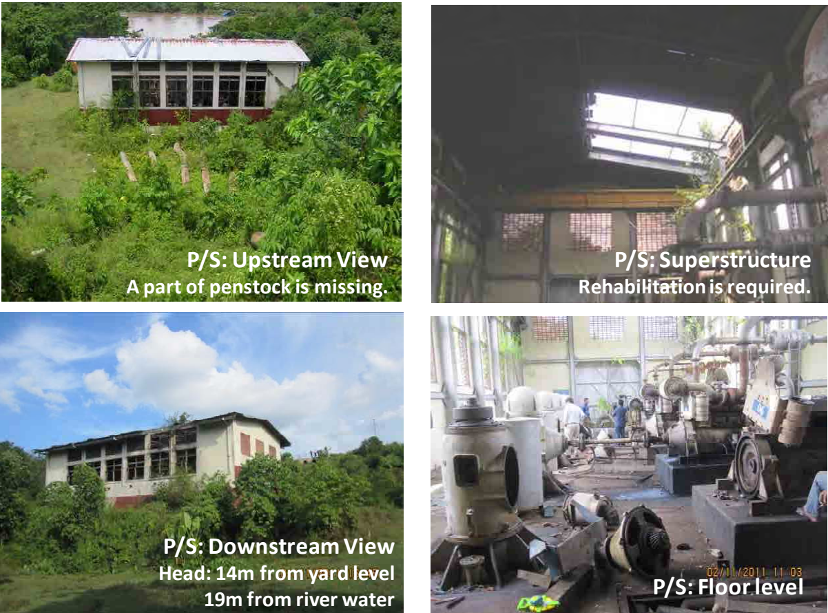
Figure 5.3.3 SEDASI Pump Station
