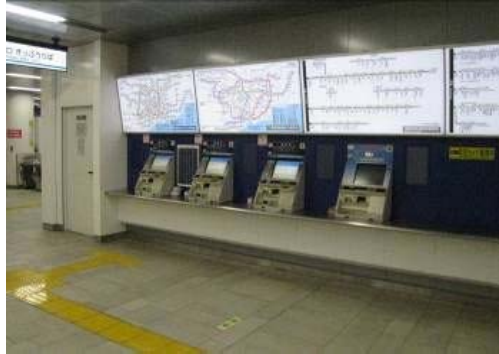
Photo 2.3.3.9-2 Automatic Ticket Machine and Charger
