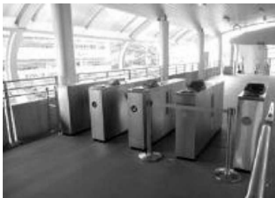
Ticketing turnstiles at entry exit to a prepaid platform area (Bangkok BRT)
