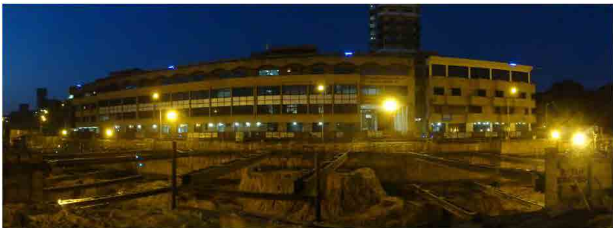
(d) Nightly view of HAL building and the excavation site Figure 3.13 Installation of tilt meters on HAL building
