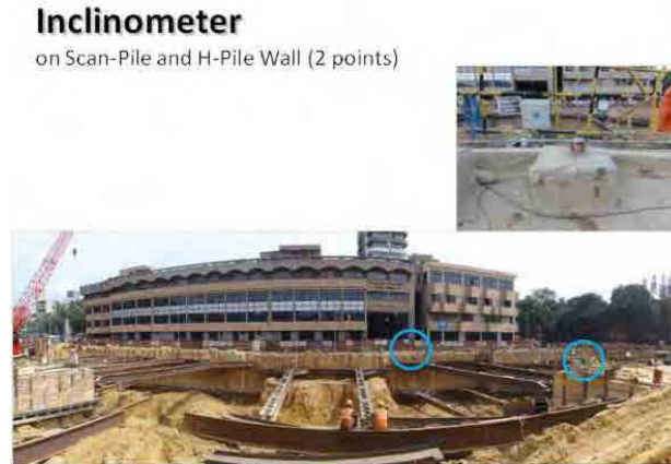
(a) Two locations (in blue circles) where multiple inclination sensors were installed
