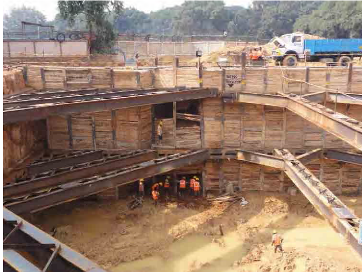
Figure 3.24 Loss of soil behind the wall on the south side of Cricket Stadium station
