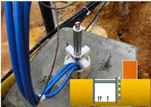
(b) Top of a casing pipe for inclination sensors
