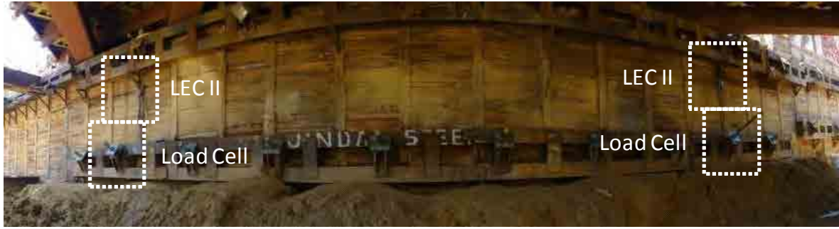
(a) Location for anchor force monitoring
