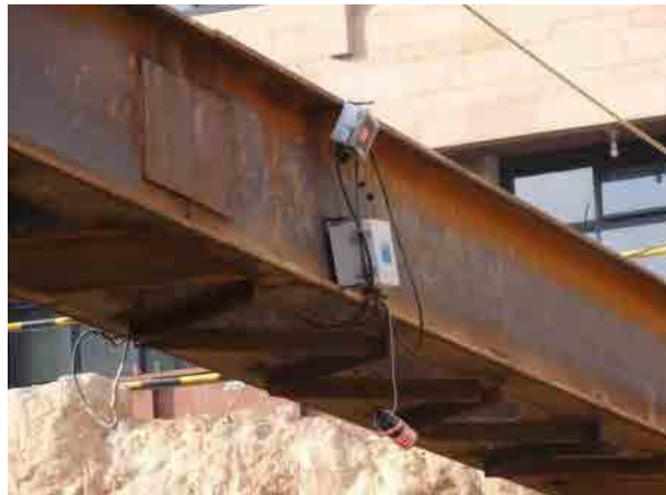
Figure 3.21 LEC showing Red due to temperature effect
