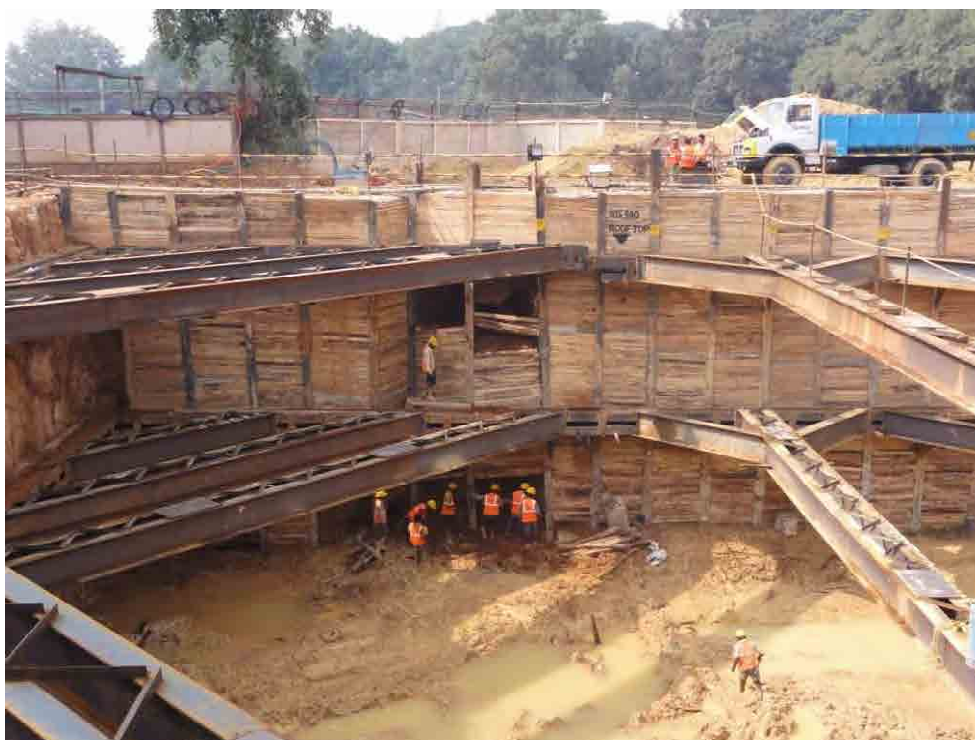
Potential problem found behind the wall where OSV sensors were not installed.
