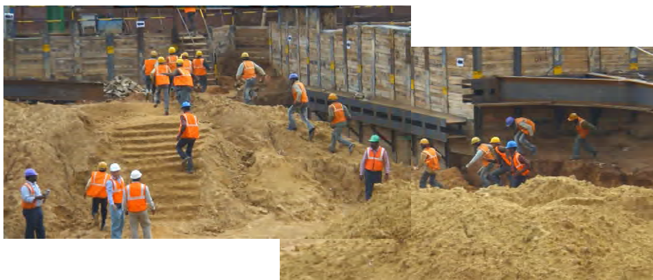
Figure 6.13 The condition before evacuation and after evacuation
