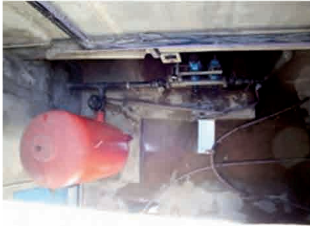
Hydropneumatical central for service water
