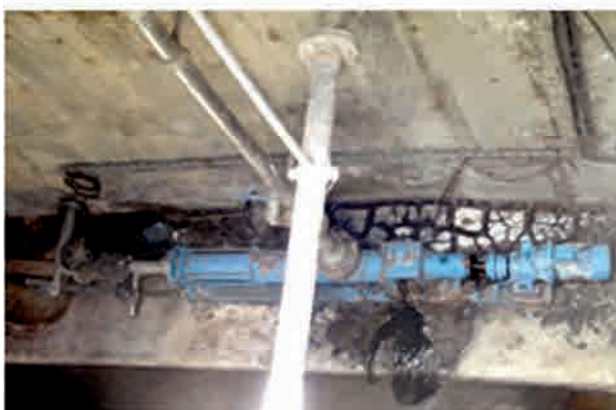
Sludge extraction pump
