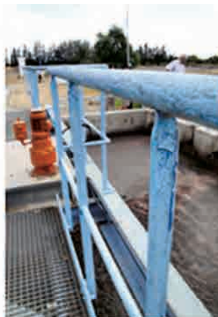
Thickener scraper bridge
