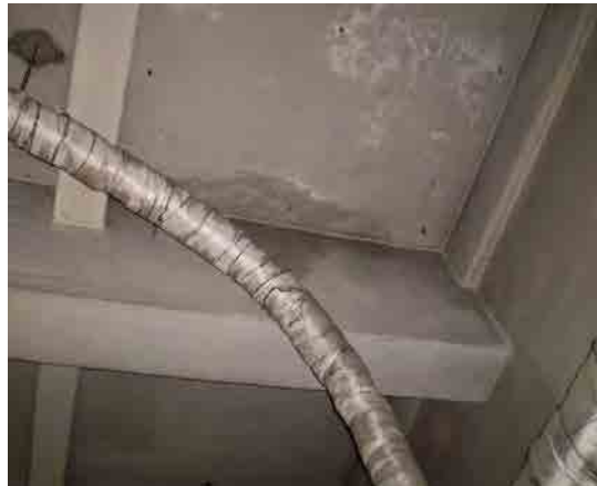
Photo 4: Parts of rain water leakage
