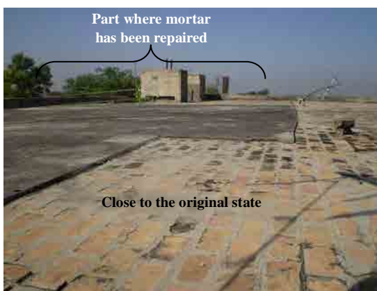
Photo 1: Conditions of the roof
