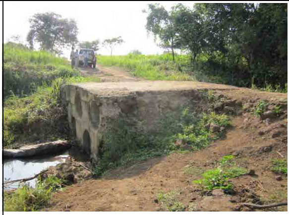
Washed out culvert due to poor construction
