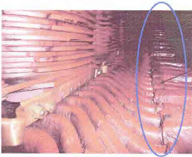
Photo-1: 2G4 Insulation caps at WT side
