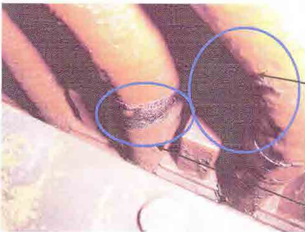
Photo-2: 2G4 Field coil (Interpole) and stator coil ends
