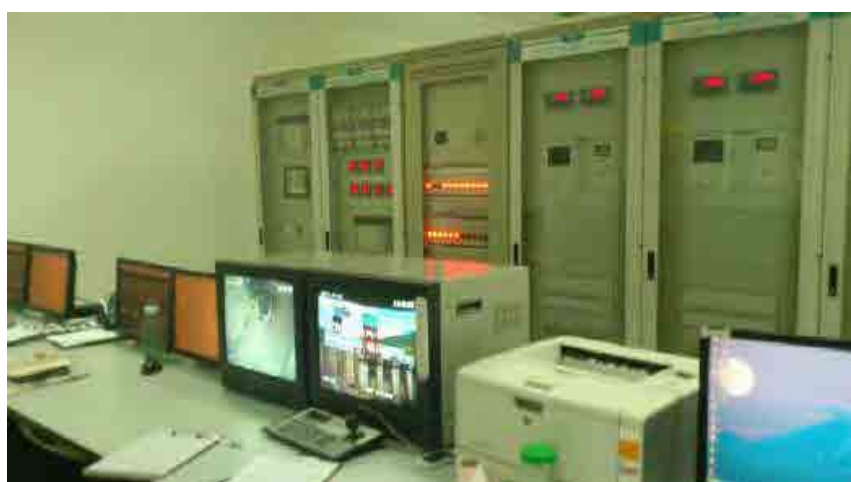
Figure 13 Control room of PH2
