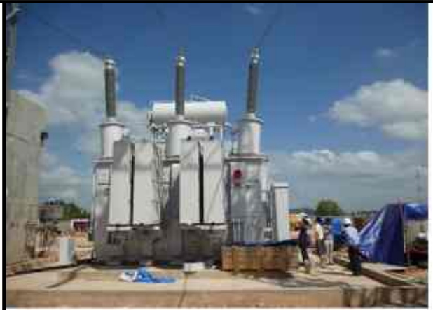
Transformer (230/22kV, 50MVA)
