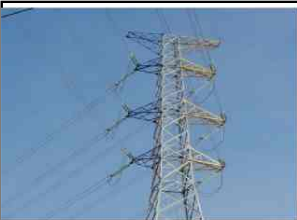
230kV Transmission line (Left: Blue colored, Right: Yellow colored) Insulators made of glass
