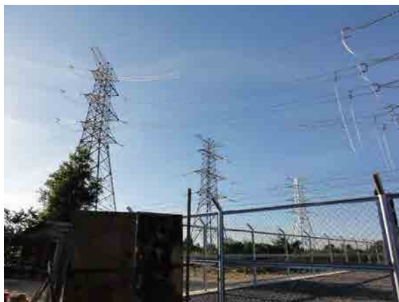
Figure 8 Towers (left: to Phnom Penh, middle: to O'soam, right: to Battambang)
