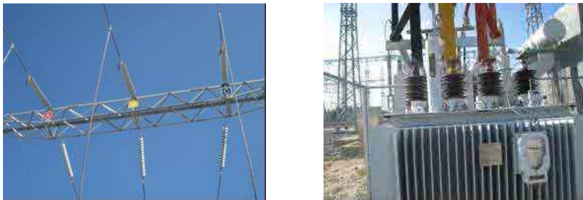
Figure 2 Phase signs on outdoor structure and facility
