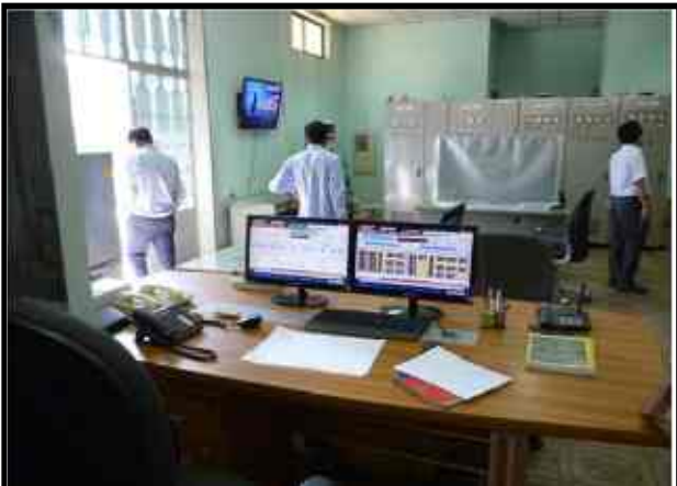
Control Room of GS3
