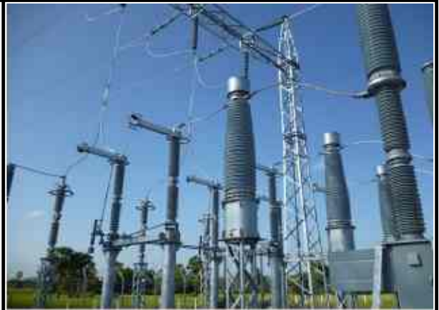
Circuit Breaker and Disconnecting Switch
