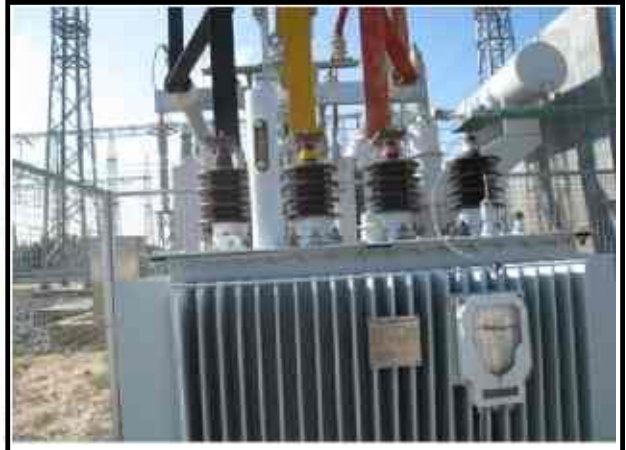
Phase Sign of Transformer
