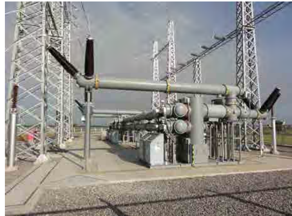
Figure 2 115kV Circuit (Gas Insulated Switch)
