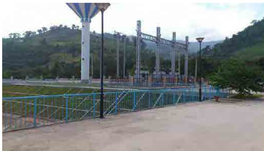
Figure 12 Switchyard of PH2
