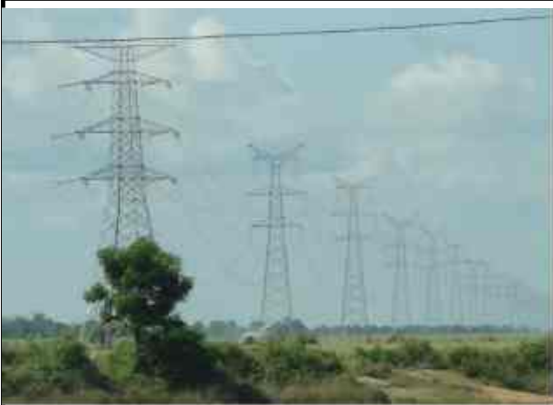
230kV Transmission Line between Battambang and Pursat
