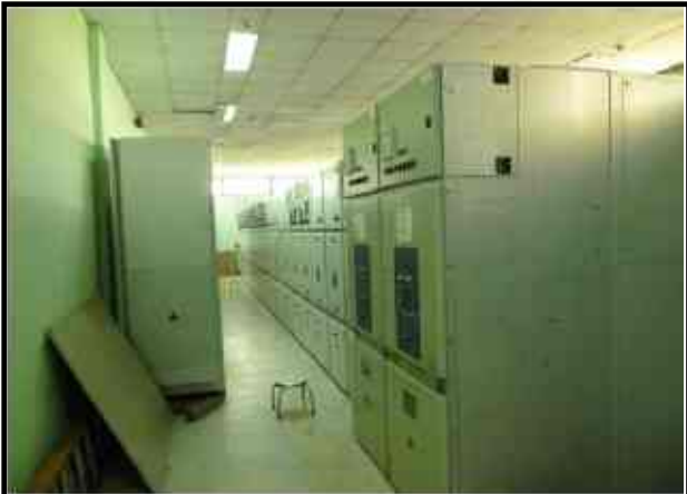
22kV Switch Gear in GS2
