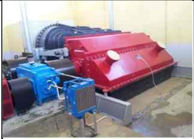
Water Turbine, Anlog Chrey Hydropower Project, Krang Ponley Irrigation Project
