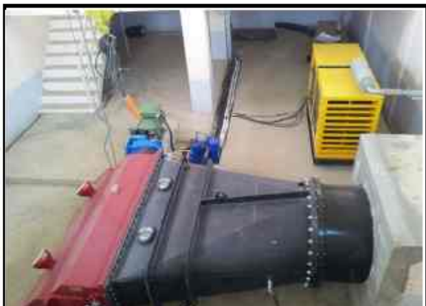
Waterturbine, Krapeu Truom Hydropower Project, Krang Ponley Irrigation Project
