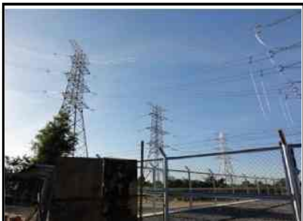
Pursat GS (Left tower: to Kampong Chhunang GS, Middle: to O'soam GS, Right: to Battambang GS)
