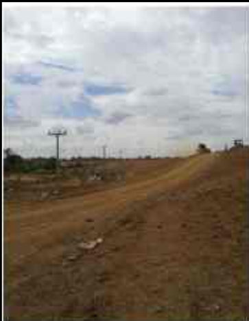
Earth Dam & Transmission Line Powerhouse and Dam Spillway, Anlog Chrey Hydropower Project, Krang Ponley Irrigation Project
