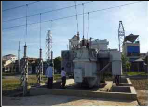
Transformer in GS1 (115/22kV, 50MVA)
