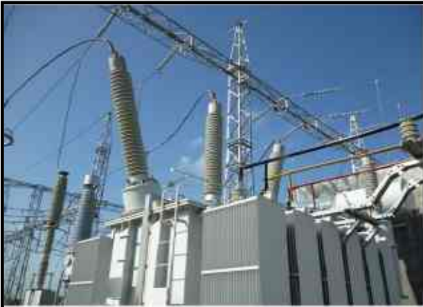
Transformer (230/22kV, 16MVA)
