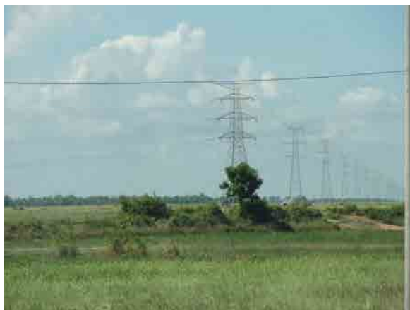
Figure 3 230kV Transmission Line
