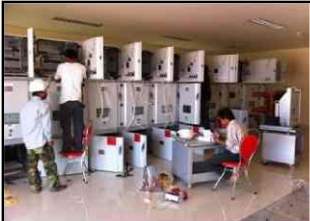
22kV Switch Gear
