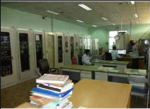
Control Room of GS1
