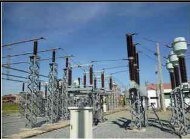
Equipment of Grid Substation 2
