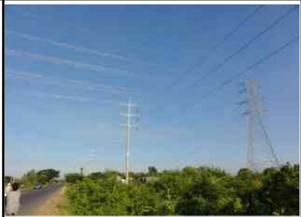
115kV Transmission Line and 230kV Transmission Line near Battambang GS
