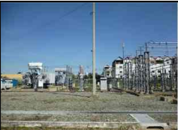
Equipment of Grid Substation 3
