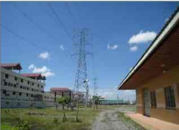
Nov. 23, 2011 Transmission Line Training Tower at EDC Training Center
