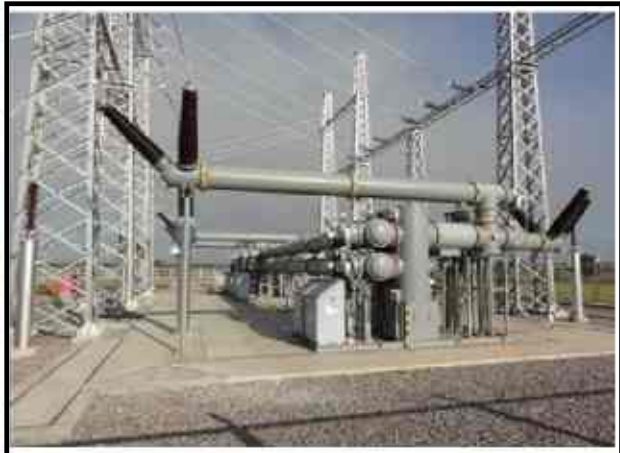
115kV GIS Switchgear at Battambang GS
