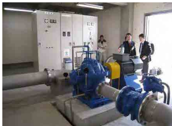
Pump reverse running turbine (Kawasaki Plant Systems experimental)
