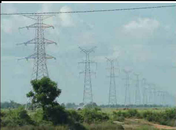
230kV Transmission Line between Battambang and Pursat
