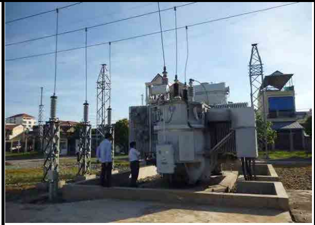
Transformer in GS1 (115/22kV, 50MVA)
