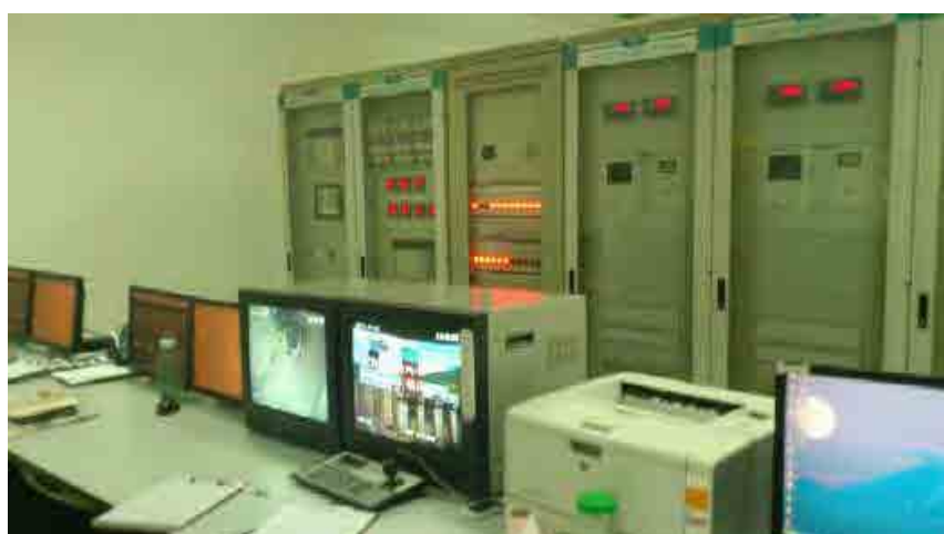
☒ 13 Control room of PH2
