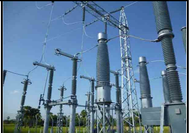
Circuit Breaker and Disconnecting Switch
