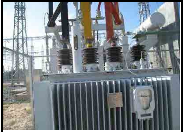
Phase Sign of Transformer
