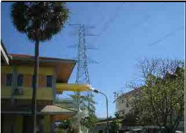
Nov. 23, 2011 Transmission Line Training Tower at EDC Training Center
