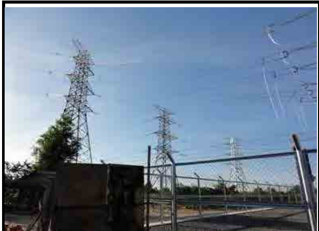
Pursat GS (Left tower: to Kampong Chhunang GS, Middle: to O'soam GS, Right: to Battambang GS)
