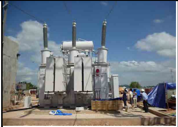
Transformer (230/22kV, 50MVA)
