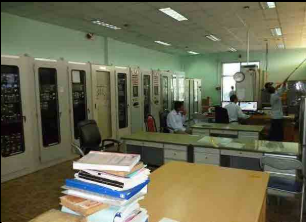
Control Room of GS1
