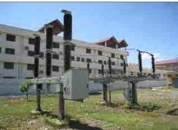
Nov. 23, 2011 Substation Training Equipment at EDC Training Center
