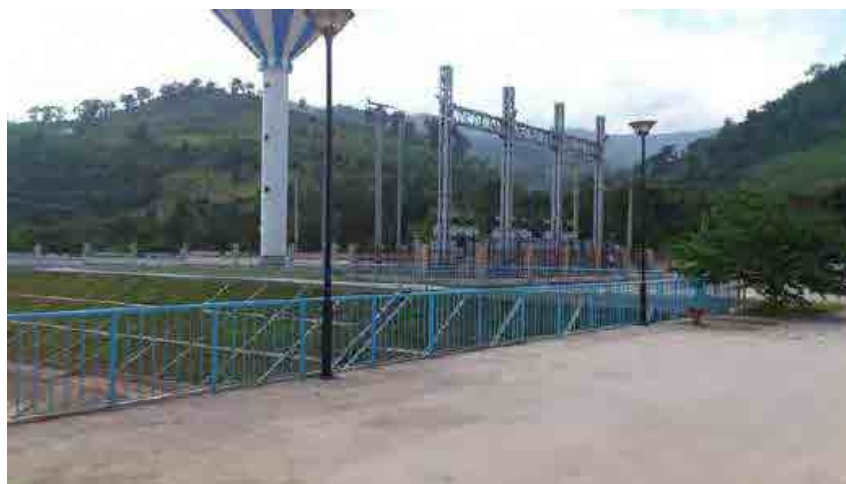
☒ 12 Switchyard of PH2
