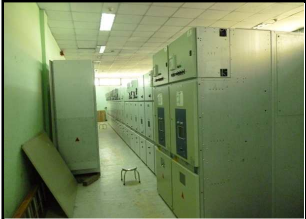
22kV Switch Gear in GS2
