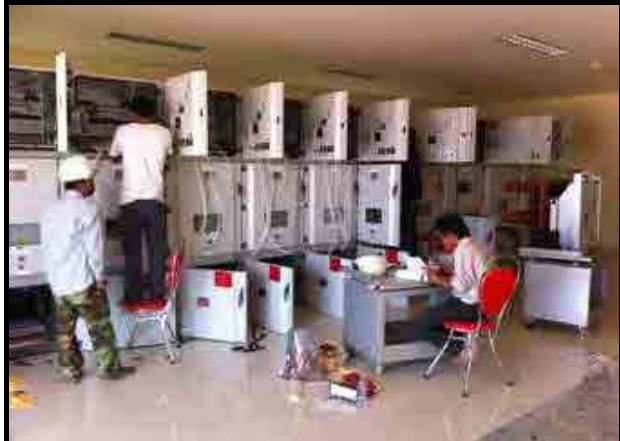
22kV Switch Gear
