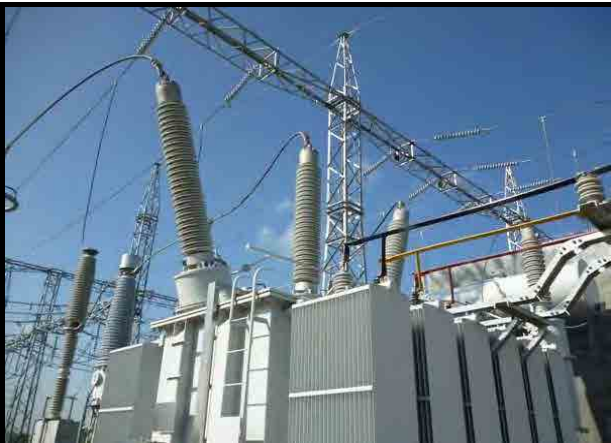
Transformer (230/22kV, 16MVA)
