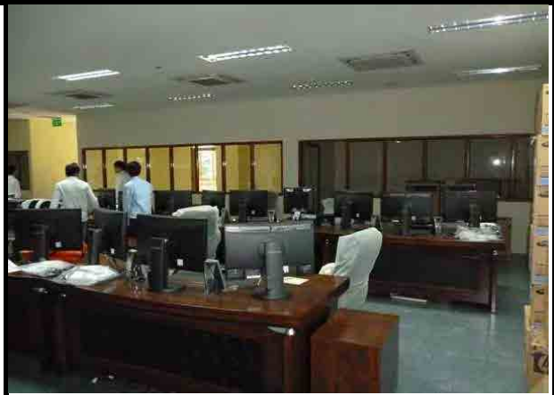
Nov. 23, 2011 Control Room of NCC
