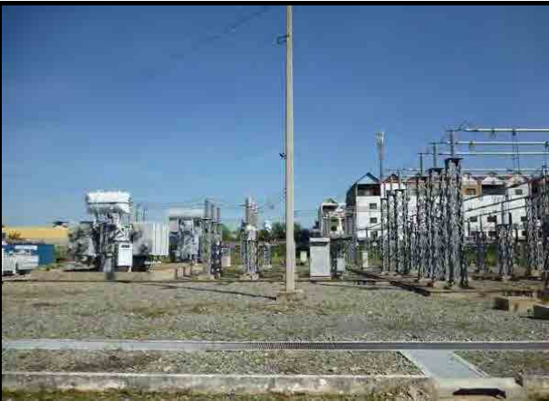
Equipment of Grid Substation 3
