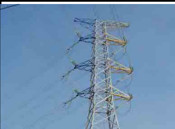
230kV Transmission line (Left: Blue colored, Right: Yellow colored) Insulators made of glass
