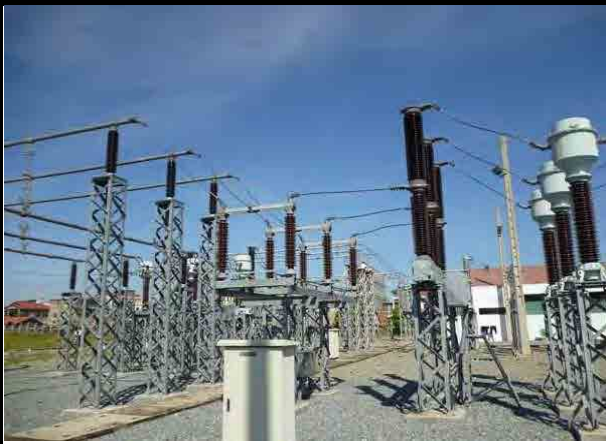
Equipment of Grid Substation 2
