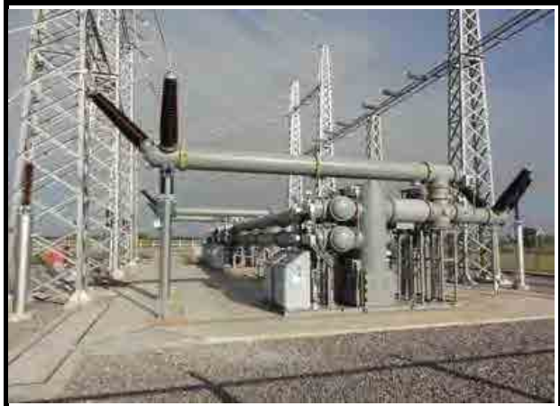
115kV GIS Switchgear at Battambang GS
