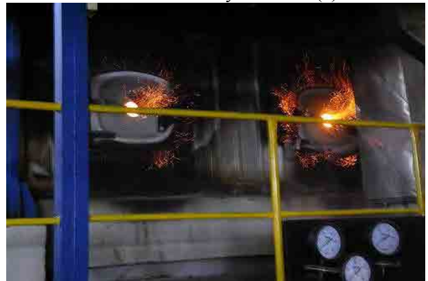
Biomass thermal energy generation
