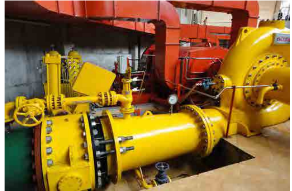
Adavikanda Mini-Hydro Power (2)
