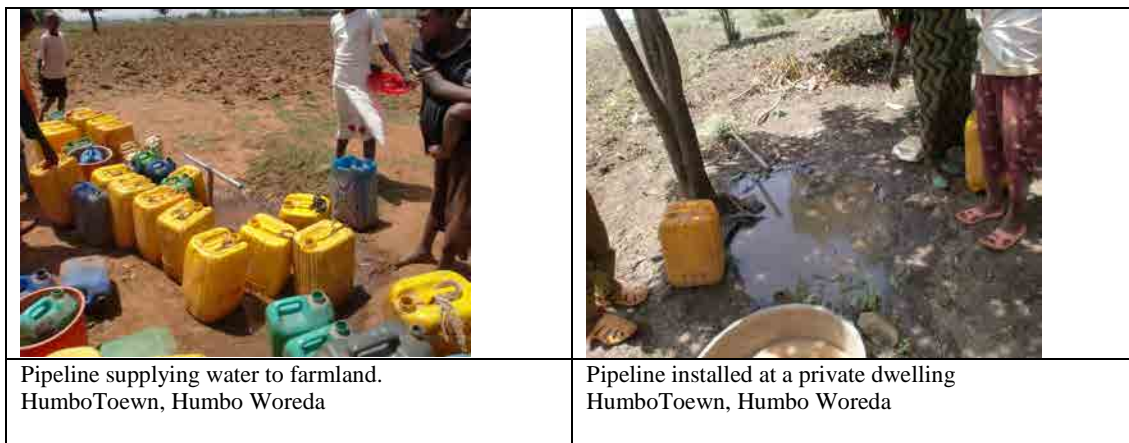
Figure 9.3: Open Pipeline Water Supply System
