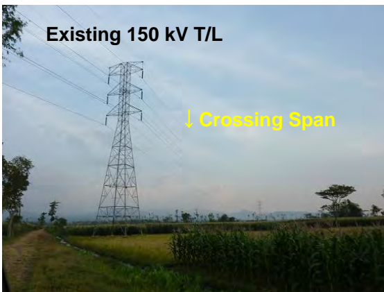
Existing 150 kV T/L crossing between T.391 and T.392
