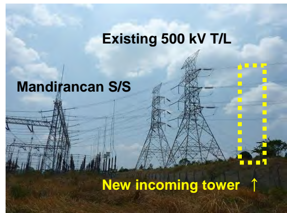
Incoming tower to Mandirancan SS
