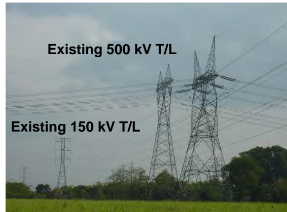
Crossing of existing 150 kV & 500 kV T/L
