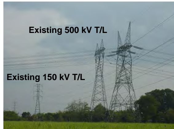
Crossing of existing 150 kV & 500 kV T/L
