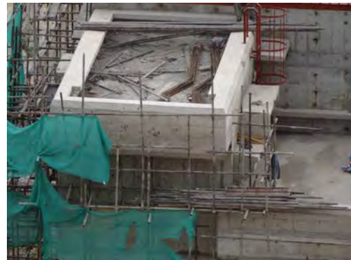
Risk in temporary work at elevated place
