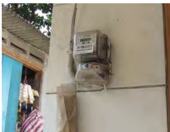
Figure 2.2.1-2 PLN's Watt-hour Meter (Measuring the Total Electricity Consumption)
