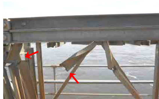
Photo-4 Damage of Existing Juba Bridge Panels due to Accident
