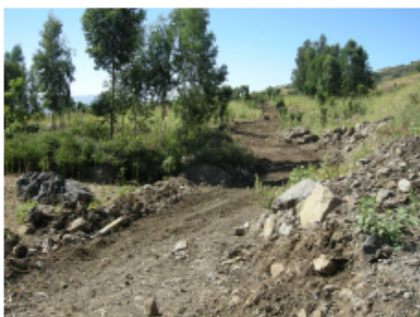
Construction of access road for drilling points B27-13 and B27-24 (maize field)
