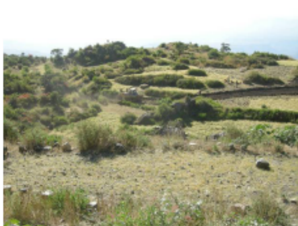
Construction of access road for drilling points B00-15 and B00-16 (teff field)
