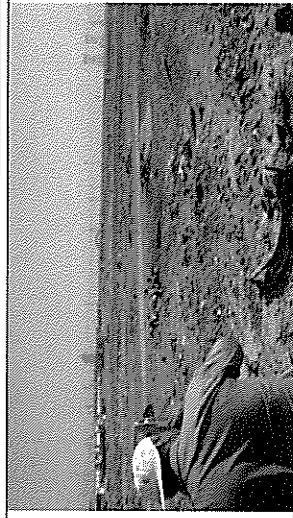
Total station and survey team surveying the plane area in front of existing power plant
