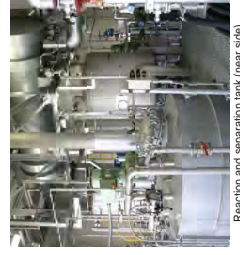
Reaction and separation tank (near side) and reaction and separated tank (far side)
