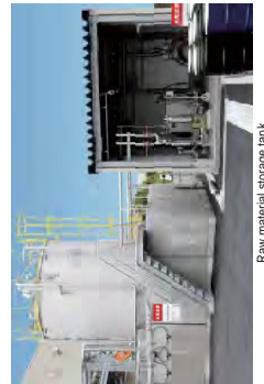
Raw material storage tank
