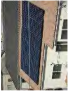
PV Panel at Local Residence generating RECs (Aichi Carbon Offsetting Association)
