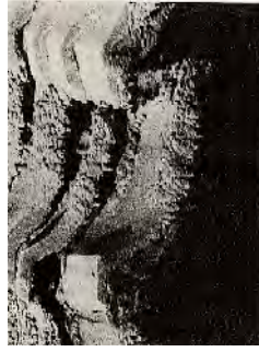
Soot and dust on the roof
