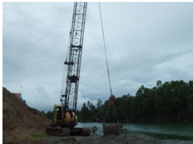
Photo 5.4.2.3.3 Limestone loading equipment
