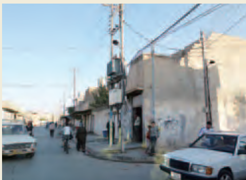
Equipment for distribution of electricity, provided via an ODA Loan (Erbil, northern part of Iraq (Kurdistan region))
