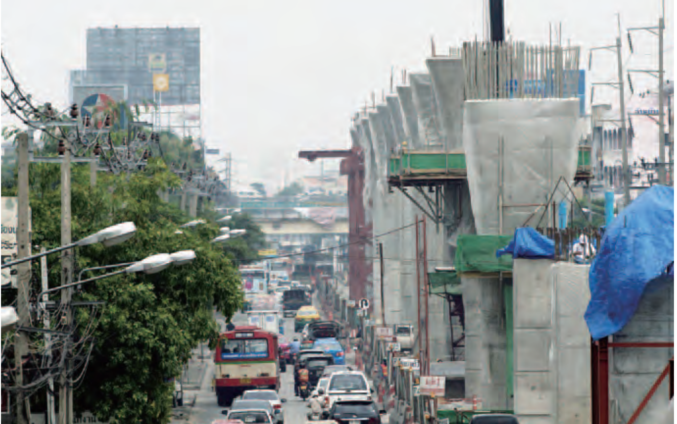
In the capital city of Bangkok, Thailand, the purple line of the mass transit system, connecting Bangkok and the neighboring Nonthaburi Province, is being constructed with the provision of ODA Loans.
