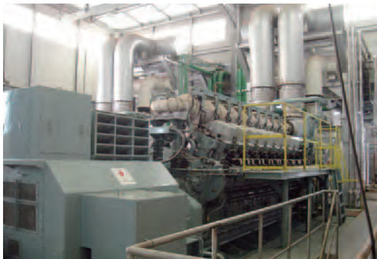
A diesel generator provided to Sierra Leone, where civil war came to an end in 2002, via Grant Aid as a means of supporting the country's economic reconstruction. JICA has provided cooperation since 2010, when the generator began operating, in order to improve Sierra Leone's capacity to operate and manage electric power facilities.
