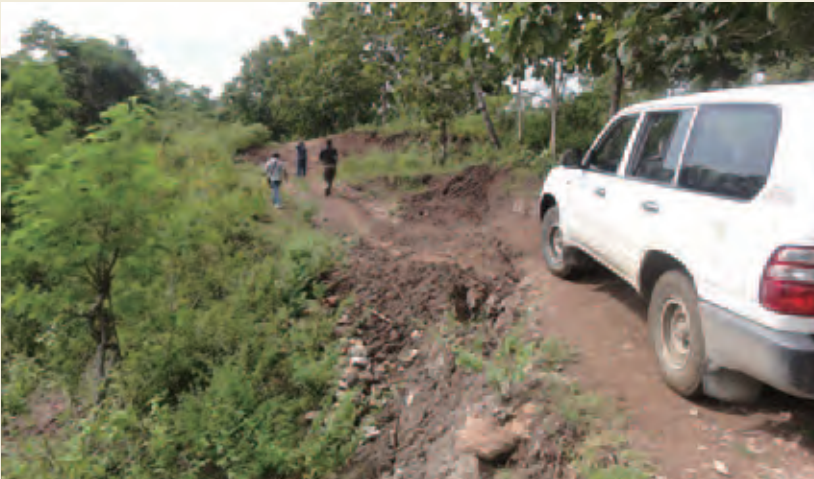
The road is continuously slanted. Coupled with the effects of heavy rain, road conditions are extremely poor.
