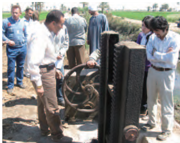
Conduit repair work at a pilot site being carried out together with an irrigation association (Water Management Improvement Plan Phase II in Egypt).
