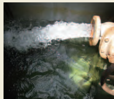
Treating water at the slow sand filtration plant
