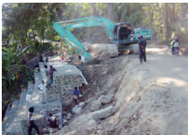
Roads are frequently blocked due to road surface damages from heavy rainfall during the rainy season (photo is of the Government’s restoration work). JICA supports capacity building in road maintenance work (Timor-Leste).
