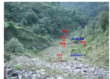
Pit1,2 : set up the Gabion2 where cobbles of Dmax300mm or more are distributed on slope ground surface Pit3,4 : set between Gabion2 and Gabion 3 Pit5,6 : set at toe-of slope of counterweight fill
