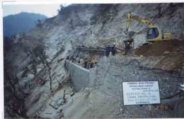
Photo No. 13 DATE : 18 February 2003 DESCRIPTION : Construction of Reinforced Earth Wall LOCATION : Sta. 17+521-17+582
