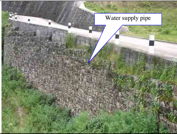
Water supply pipe within the location of the planned anchor installation (need to be removed)
