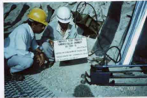
Photo No. 19 DATE : 05 March 2003 DESCRIPTION : Reinforced Earth Wall - B Anchor Pulling Test Inspection by the Consultant LOCATION : Sta. 17+620-17+648
