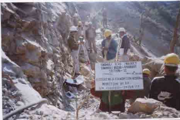
Photo No. 14 DATE : 12 January 2003 DESCRIPTION : Reinforced Earth Wall - B Foundation Bedding Inspection by the Consultant LOCATION : Sta. 17+549-17+558
