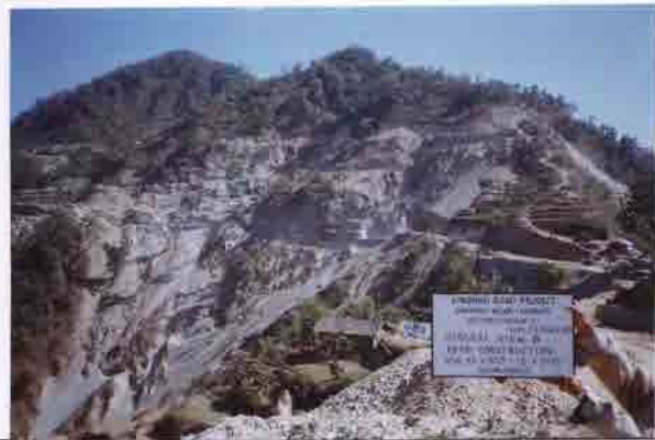
Photo No. 7 DATE : 20 January 2003 DESCRIPTION : General View of Road Construction LOCATION : Sta. 17+400-18+300
