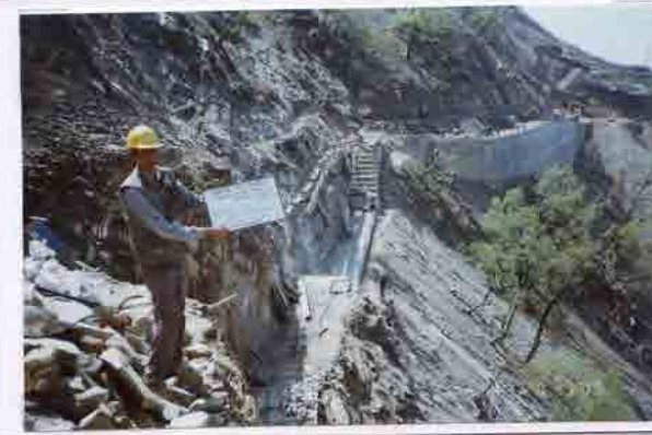
Photo No. 11 DATE : 20 March 2003 DESCRIPTION : General View of Road Construction LOCATION : Sta. 17+650-17+500
