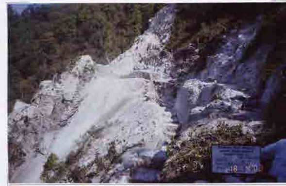
Photo No. 14 DATE : 18 April 2003 DESCRIPTION : General View of Road Construction LOCATION : Sta. 19+550-19+750
