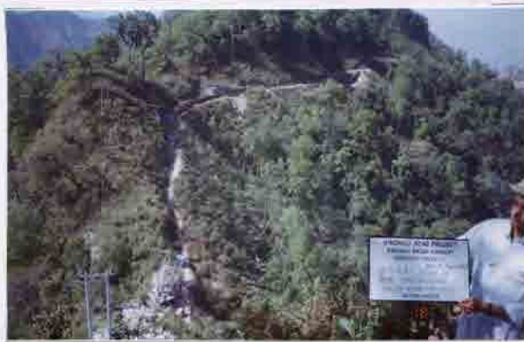
Photo No. 12 DATE : 18 April 2003 DESCRIPTION : General View of Road Construction LOCATION : Sta. 19+300-19+000
