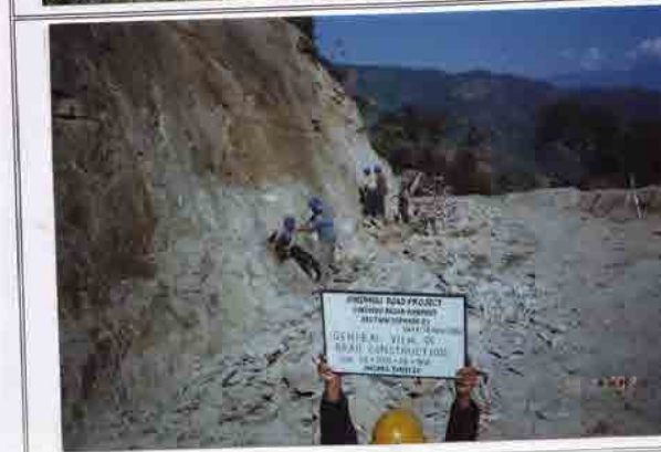
Photo No. 6 DATE : 18 November 2002 DESCRIPTION : General View of Road Construction LOCATION : Sta. 19+900-20+900
