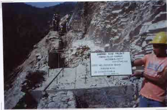
Photo No. 19 DATE : 06 May 2003 DESCRIPTION : Gabion Wall Foundation Bedding Inspection by the Consultant. LOCATION : Sta. 17+738-17+745
