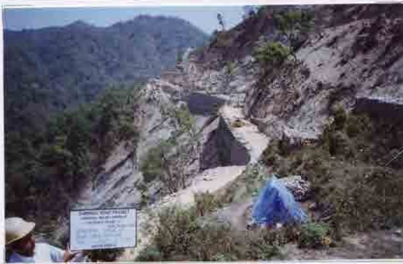
Photo No. 11 DATE : 18 April 2003 DESCRIPTION : General View of Road Construction LOCATION : Sta. 17+500-17+700
