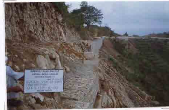
Photo No. 10 DATE : 15 June 2003 DESCRIPTION : General View of Road Construction LOCATION : Sta. 16+577-16+660
