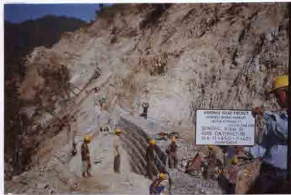
Photo No. 8 DATE : 20 January 2003 DESCRIPTION : General View of Road Construction LOCATION : Sta. 17+450-17+600
