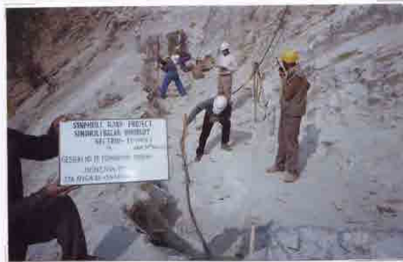
Photo No. 14 DATE : 14 February 2003 DESCRIPTION : Reinforced Earth Wall Foundation Inspection by the Consultant LOCATION : Sta. 17+620-17+646
