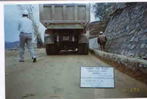
Photo No. 21 DATE : 14 March 2003 DESCRIPTION : Road Pavement - Sub-Grade Proof Rolling Inspection by the Consultant LOCATION : Sta. 16+500-17+000
