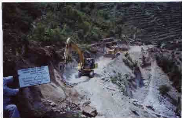
Photo No. 21 DATE : 10 May 2003 DESCRIPTION : Construction of Temporary Access Road LOCATION : Sta. 18+650-17+850
