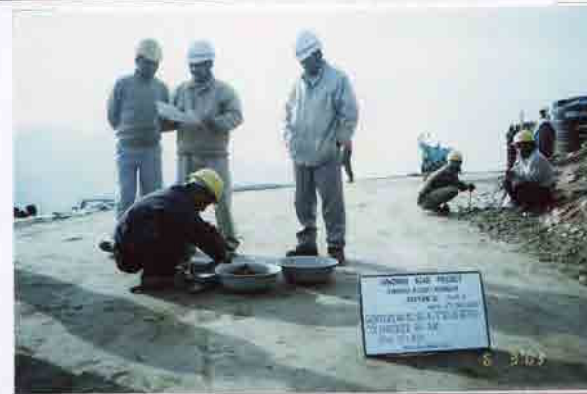
Photo No. 20 DATE : 06 March 2003 DESCRIPTION : Reinforced Earth Wall - A Field Density Inspection by the Consultant LOCATION : Sta. 15+850
