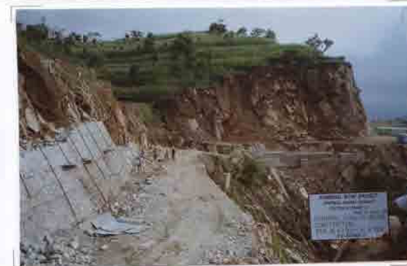
Photo No. 11 DATE : 15 June 2003 DESCRIPTION : General View of Road Construction LOCATION : Sta. 16+750-16+700
