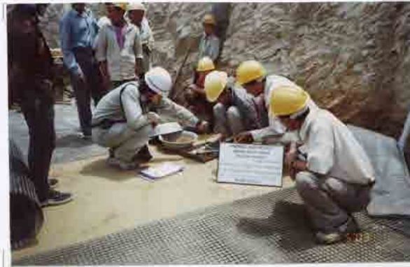
Photo No. 20 DATE : 09 May 2003 DESCRIPTION : Reinforced Earth Wall - B 8th Layer Field Density Inspection by the Consultant LOCATION : Sta. 17+706-17+719
