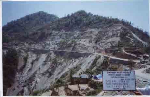
Photo No. 10 DATE : 18 April 2003 DESCRIPTION : General View of Road Construction LOCATION : Sta. 17+400-18+300
