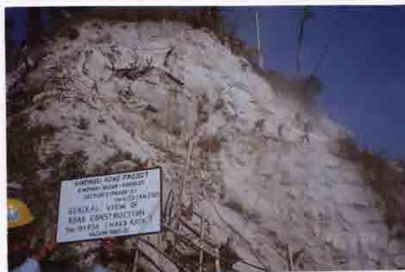
Photo No. 9 DATE : 20 January 2003 DESCRIPTION : General View of Road Construction LOCATION : Sta. 19+950
