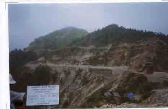
Photo No. 12 DATE : 15 June 2003 DESCRIPTION : General View of Road Construction LOCATION : Sta. 17+400-18+300
