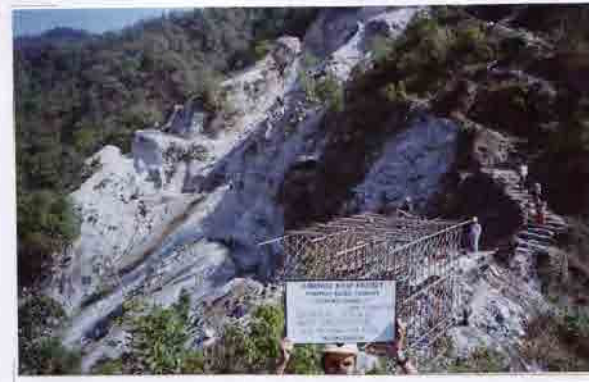
Photo No. 13 DATE : 18 April 2003 DESCRIPTION : General View of Road Construction LOCATION : Sta. 19+400-19+500
