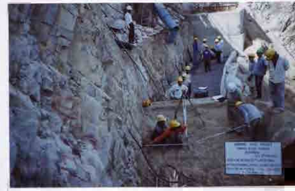
Photo No. 15 DATE : 16 April 2003 DESCRIPTION : Reinforced Earth Wall 1st Layer Panel Setting, Geo Grid Laying & Gabion Bedding Inspection by the Consultant LOCATION : Sta. 17+706-17+719
