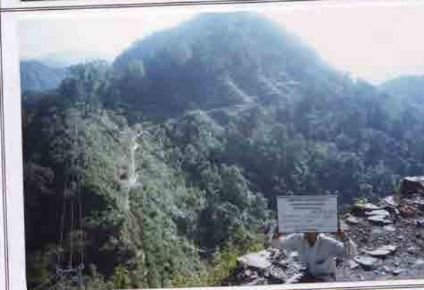
Photo No. 5 DATE : 18 November 2002 DESCRIPTION : General View of Road Construction LOCATION : Sta. 19+300-19+400
