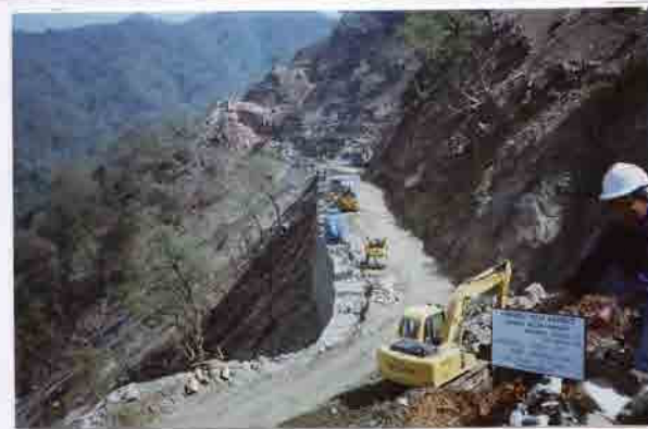
Photo No. 10 DATE : 29 March 2003 DESCRIPTION : General View of Road Construction LOCATION : Sta. 17+500-17+700
