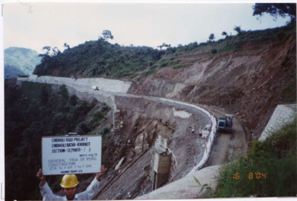
Photo No. 8 DATE : 16 August 2004 DESCRIPTION : General View of Road Construction LOCATION : Sta. 16+025-16+200
