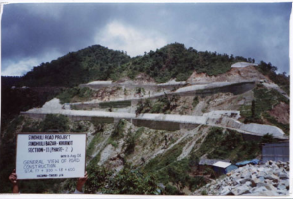
Photo No. 9 DATE : 16 August 2004 DESCRIPTION : General View of Road Construction LOCATION : Sta. 17+300-18+600
