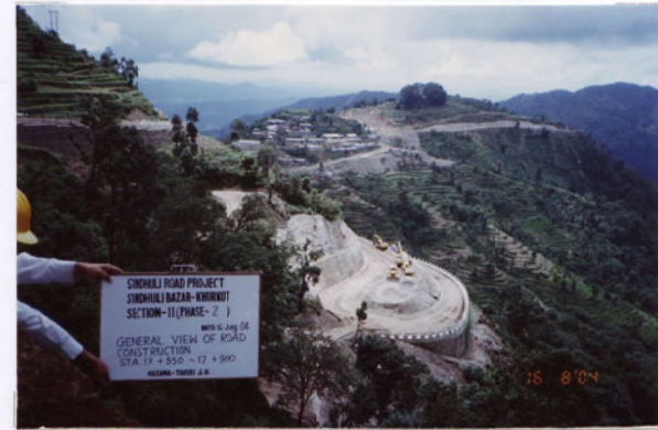
Photo No. 10 DATE : 16 August 2004 DESCRIPTION : General View of Road Construction LOCATION : Sta. 17+950-17+900
