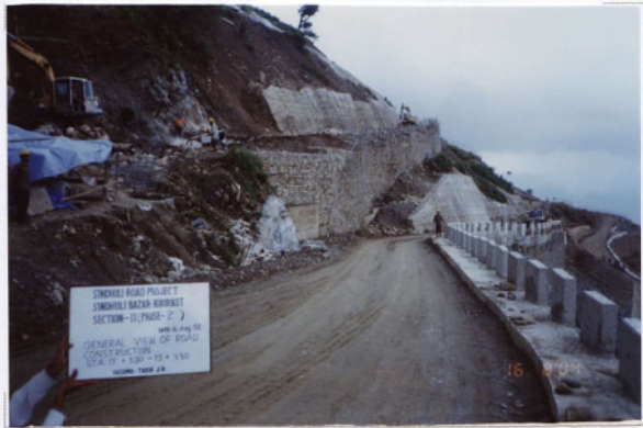
Photo No. 7 DATE : 16 August 2004 DESCRIPTION : General View of Road Construction LOCATION : Sta. 15+530-15+330
