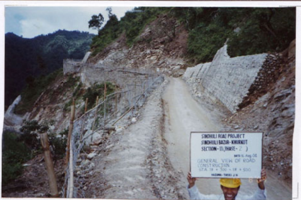
Photo No. 12 DATE : 16 August 2004 DESCRIPTION : General View of Road Construction LOCATION : Sta. 18+300-18+500
