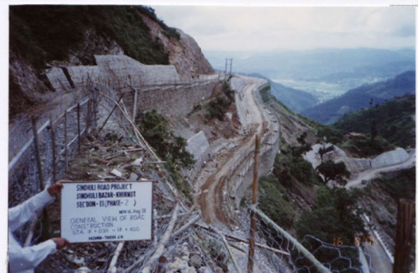
Photo No. 11 DATE : 16 August 2004 DESCRIPTION : General View of Road Construction LOCATION : Sta. 18+030-18+400
