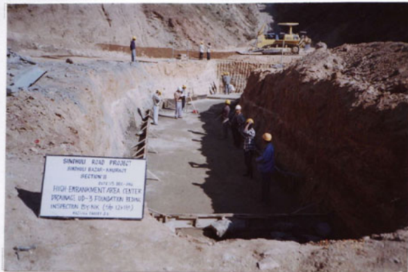
Photo No. 10 DATE : 15 December 2002 DESCRIPTION : High Embankment - Center Drainage UD-3 Foundation Bedding Inspection by the Consultant LOCATION : Sta. 12+180
