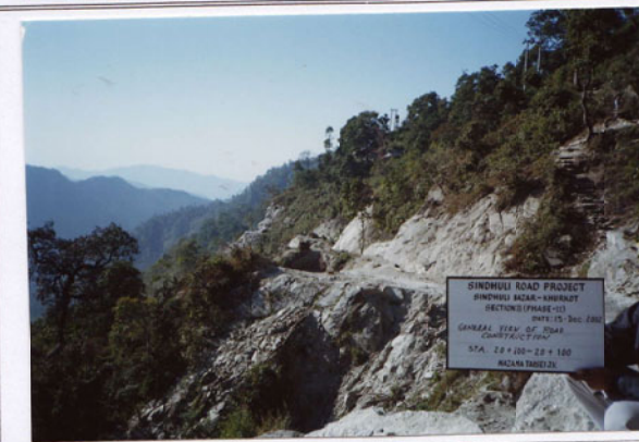
Photo No. 6 DATE : 15 December 2002 DESCRIPTION : General View of Road Construction LOCATION : Sta. 20+100-20+100
