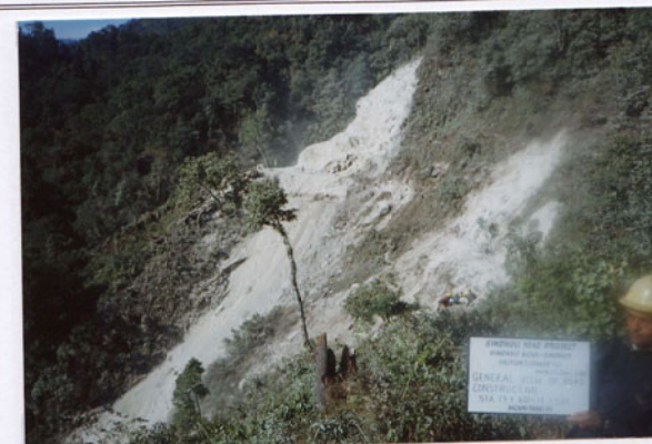
Photo No. 5 DATE : 15 December 2002 DESCRIPTION : General View of Road Construction LOCATION : Sta. 19+400-19+500
