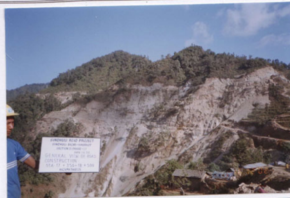
Photo No. 4 DATE : 16 December 2002 DESCRIPTION : General View of Road Construction LOCATION : Sta. 17+350-18+500
