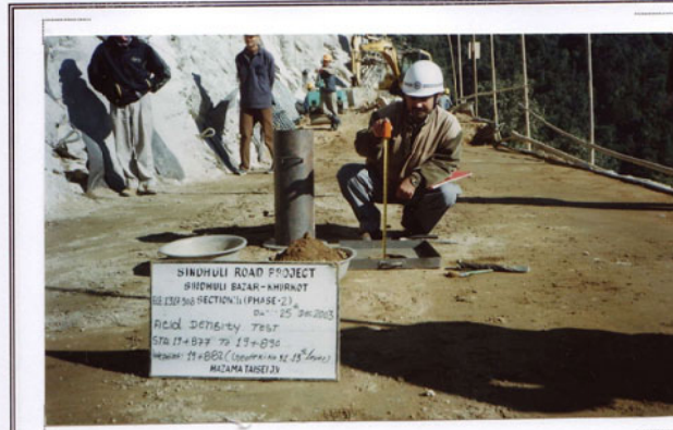
Photo No. 25 DATE : 25 December 2003 DESCRIPTION : Reinforced Earth Wall - "B" Field Density Inspection by the Consultant LOCATION : Sta. 19+877-19+890
