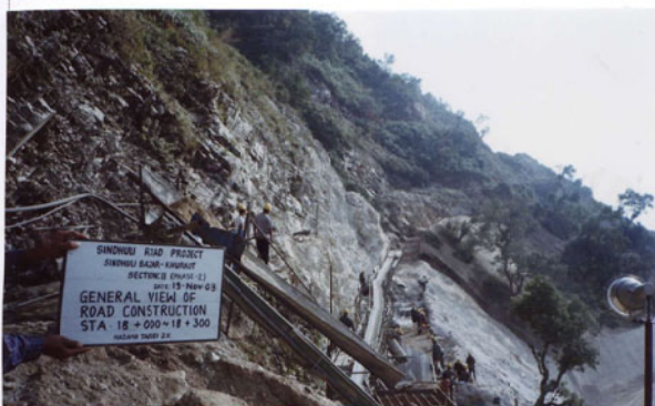
Photo No. 9 DATE : 19 November 2003 DESCRIPTION : General View of Road Construction LOCATION : Sta. 18+000-18+300
