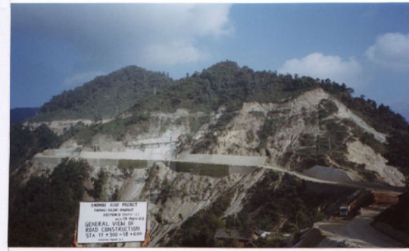
Photo No. 7 DATE : 19 November 2003 DESCRIPTION : General View of Road Construction LOCATION : Sta. 17+300-18+600
