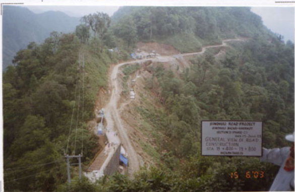
Photo No. 15 DATE : 15 June 2003 DESCRIPTION : General View of Road Construction LOCATION : Sta. 19+400-19+000
