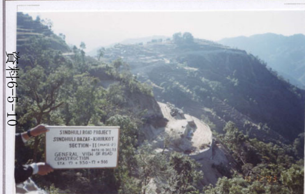
Photo No. 8 DATE : 18 December 2003 DESCRIPTION : General View of Road Construction LOCATION : Sta. 17+950-17+900
