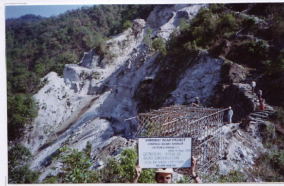
Photo No. 13 DATE : 18 April 2003 DESCRIPTION : General View of Road Construction LOCATION : Sta. 19+400-19+500
