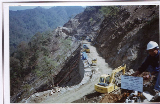
Photo No. 10 DATE : 20 March 2003 DESCRIPTION : General View of Road Construction LOCATION : Sta. 17+500~17+700
