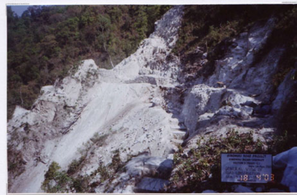
Photo No. 14 DATE : 18 April 2003 DESCRIPTION : General View of Road Construction LOCATION : Sta. 19+550-19+750
