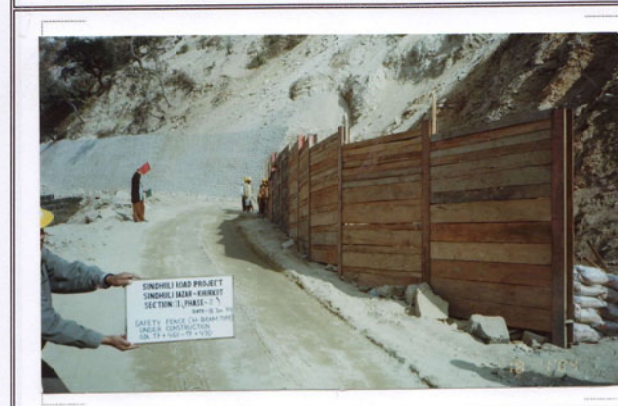
Photo No. 27 DATE : 18 January 2004 DESCRIPTION : Safety Fence (H-Beam Type) Under Construction LOCATION : Sta. 17+460-17+490
