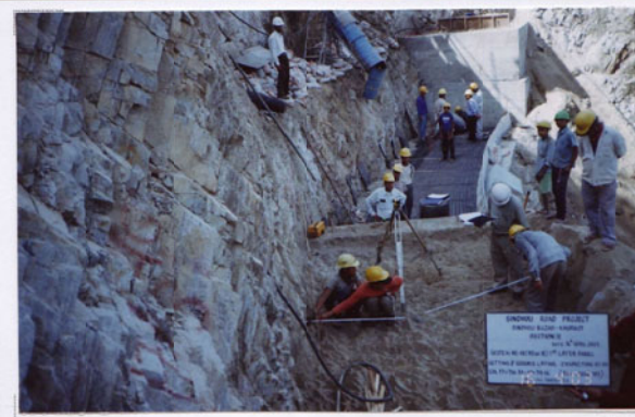
Photo No. 15 DATE : 16 April 2003 DESCRIPTION : Reinforced Earth Wall 1st Layer Panel Setting, Geo Grid Laying & Gabion Bedding Inspection by the Consultant LOCATION : Sta. 17+706-17+719
