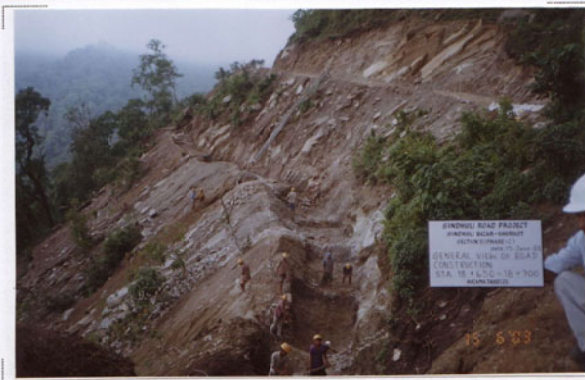
Photo No. 14 DATE : 15 June 2003 DESCRIPTION : General View of Road Construction LOCATION : Sta. 18+650-18+700
