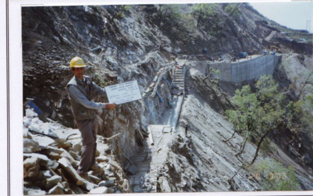
Photo No. 11 DATE : 20 March 2003 DESCRIPTION : General View of Road Construction LOCATION : Sta. 17+650~17+500
