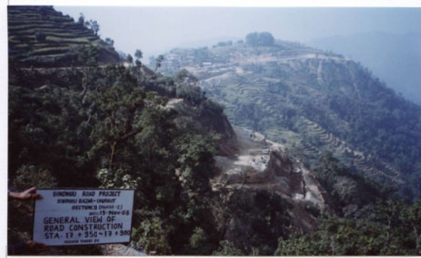
Photo No. 8 DATE : 19 November 2003 DESCRIPTION : General View of Road Construction LOCATION : Sta. 17+950-17+900
