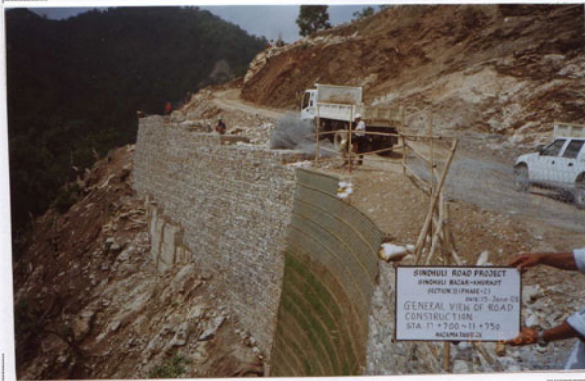
Photo No. 13 DATE : 15 June 2003 DESCRIPTION : General View of Road Construction LOCATION : Sta. 17+700-17+750
