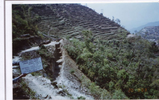
Photo No. 12 DATE : 20 March 2003 DESCRIPTION : General View of Road Construction LOCATION : Sta. 18+700~18+600
