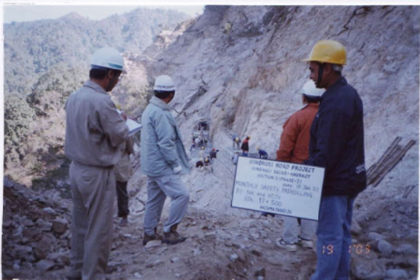
Photo No. 18 DATE : 19 January 2003 DESCRIPTION : Monthly Safety Patrolling by NK and HTJV LOCATION : Sta. 17+500
