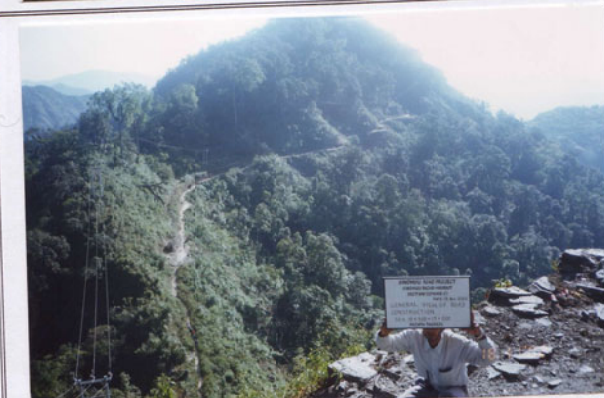
Photo No. 5 DATE : 18 November 2002 DESCRIPTION : General View of Road Construction LOCATION : Sta. 19+300-19+000
