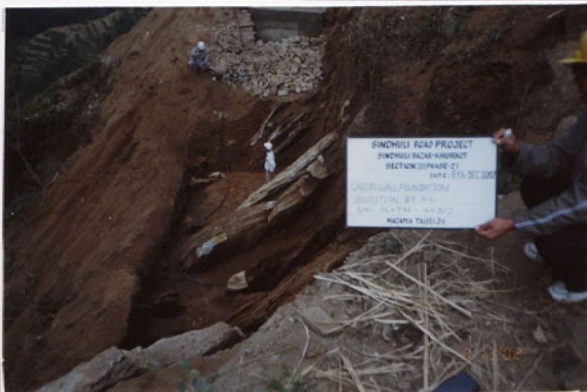
Photo No. 11 DATE : 08 December 2002 DESCRIPTION : Gabion Wall - Base Foundation Inspection by the Consultant LOCATION : Sta. 16+794-16+812
