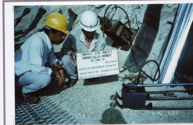
Photo No. 19 DATE : 05 March 2003 DESCRIPTION : Reinforced Earth Wall - B Anchor Pulling Test Inspection by the Consultant LOCATION : Sta. 17+620-17+648
