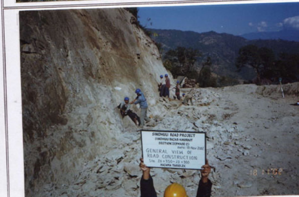
Photo No. 6 DATE : 18 November 2002 DESCRIPTION : General View of Road Construction LOCATION : Sta. 20+950-20+000
