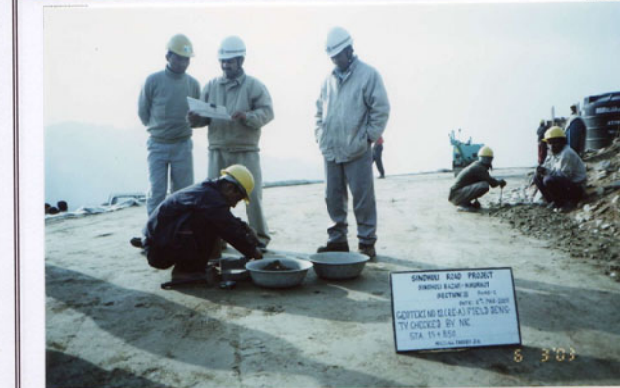
Photo No. 20 DATE : 06 March 2003 DESCRIPTION : Reinforced Earth Wall - A Field Density Inspection by the Consultant LOCATION : Sta. 15+850
