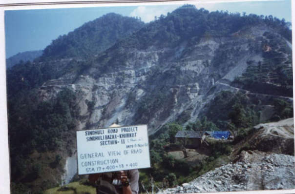
Photo No. 4 DATE : 19 November 2002 DESCRIPTION : General View of Road Construction LOCATION : Sta. 17+400-18+400
