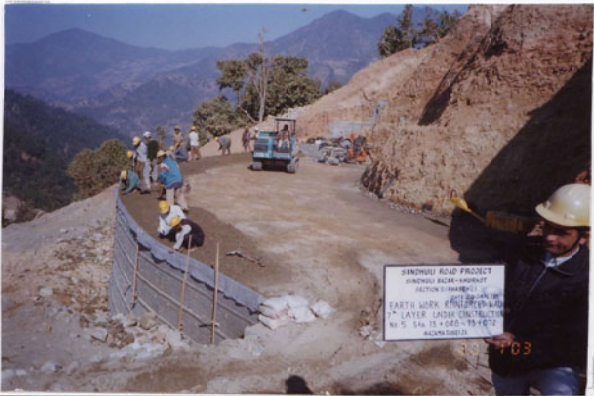
Photo No. 17 DATE : 20 January 2003 DESCRIPTION : Reinforced Earth Wall - B 7th Layer Construction LOCATION : Sta. 13+048-13+072
