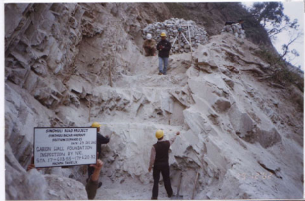
Photo No. 13 DATE : 29 December 2002 DESCRIPTION : Gabion Wall - Foundation Bedding Inspection by the Consultant LOCATION : Sta. 17+608-17+620
