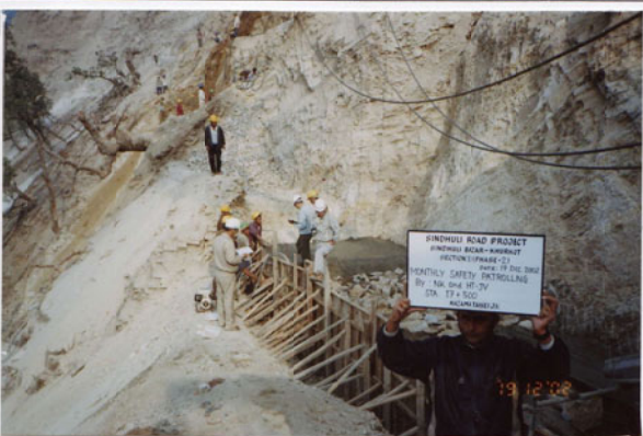
Photo No. 12 DATE : 19 December 2002 DESCRIPTION : Monthly Safety Patrolling by NK and HTJV LOCATION : Sta. 17+500
