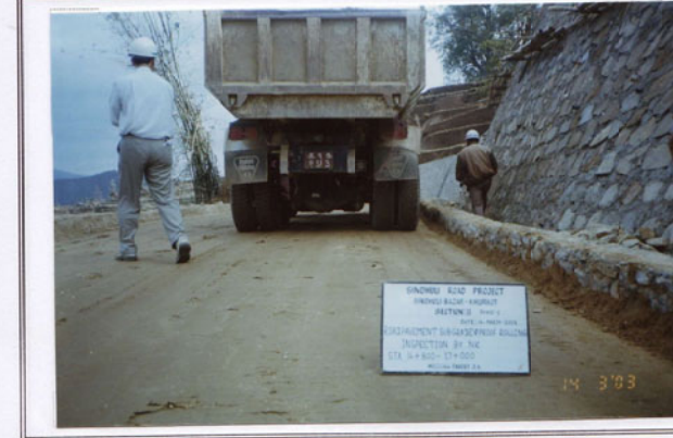
Photo No. 21 DATE : 14 March 2003 DESCRIPTION : Road Pavement - Sub Grade Proof Rolling Inspection by the Consultant LOCATION : Sta. 16+800-17+000
