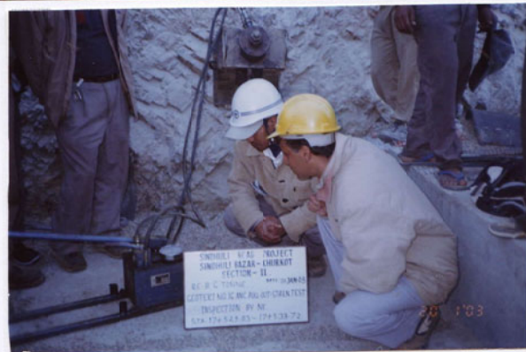
Photo No. 15 DATE : 20 January 2003 DESCRIPTION : Reinforced Earth Wall - B Anchor Pull Out Strength Test Inspection by the Consultant LOCATION : Sta. 17+529-17+533
