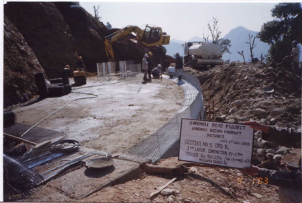
Photo No. 16 DATE : 09 January 2003 DESCRIPTION : Reinforced Earth Wall - B 3rd Layer Compaction by 1 ton Roller LOCATION : Sta. 13+048-13+072
