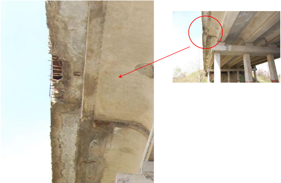
Figure 8.3.10 Deterioration of Curb (PC girder located at 90km upstream from Mykolaiv)
