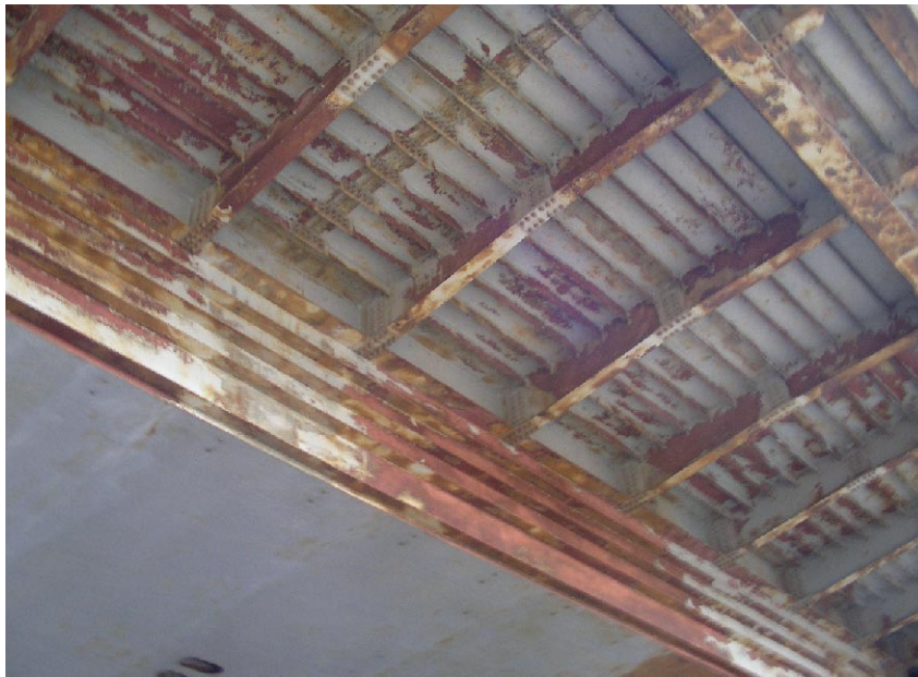
Figure 8.3.8 Corrosion of steel girder (Cable Stayed Bridge, Kiev)
