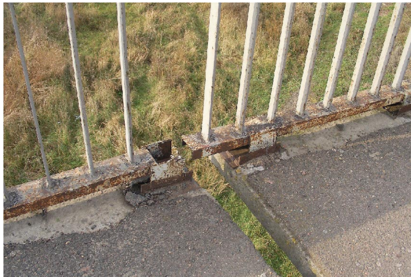
Figure 8.3.9 Deterioration/Defect of unsafe side walk (PC girder located at 90km upstream from Mykolaiv)
