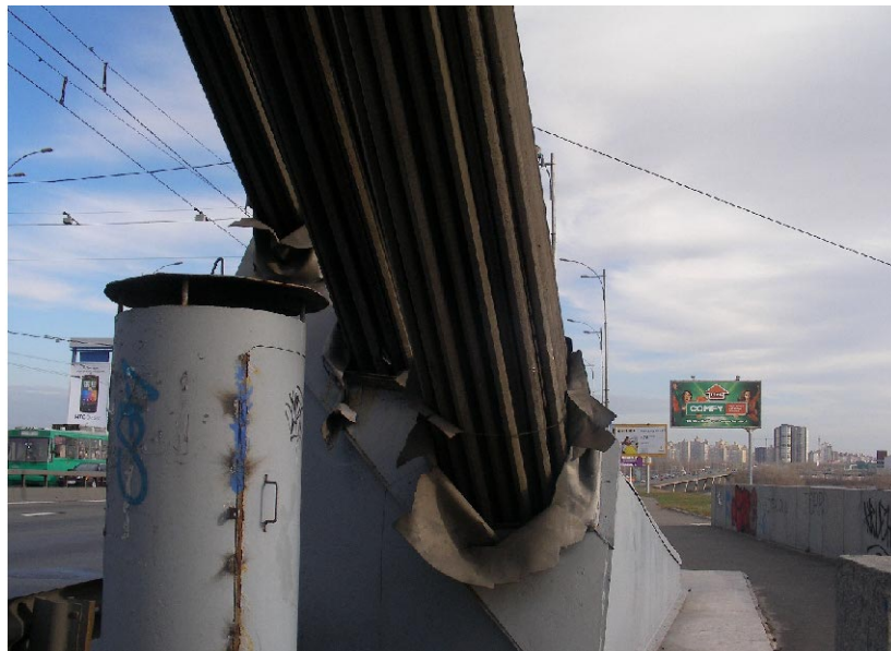
Figure 8.3.6 Breakage of waterproof cover for the stay cables (Moscow Br. Kiev)
