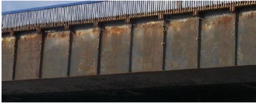
Figure 8.3.7 Corrosion of steel girder (Moscow Br. Kiev)
