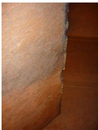
Photo-16 Trailing Edge of Wicket Gate Vane
