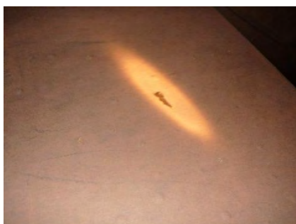
Photo-6 Stay Vane (Paint separation and water bubble is found)
