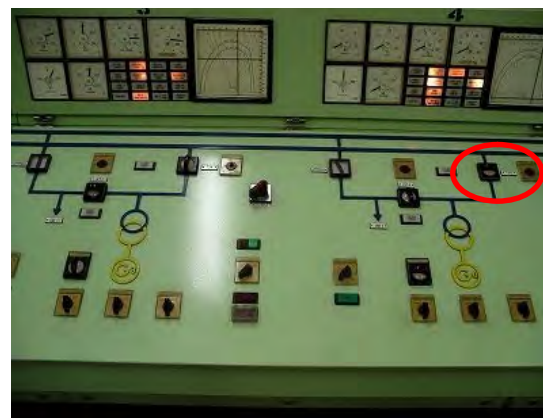
Substation Circuit Breaker Remote Control Panel (Jebba Hydroelectric Power Station Control Room)
