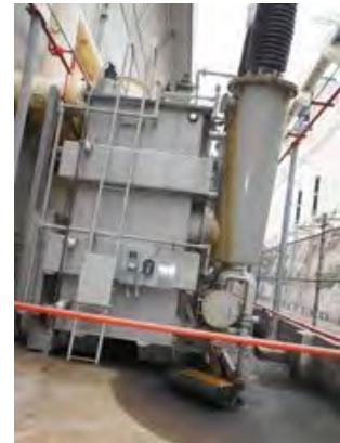
Photo 3.3-6 Oil-leaking on B phase of 2G3
