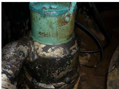
Photo-35 Drainage Pump
