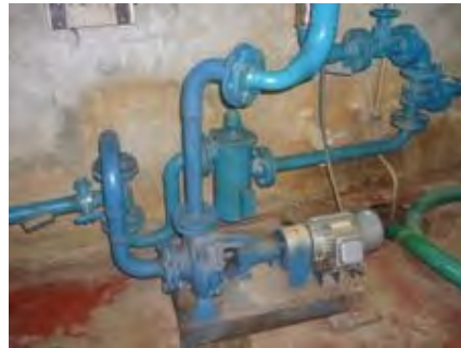
Photo 3.2-10 Water supply pump
