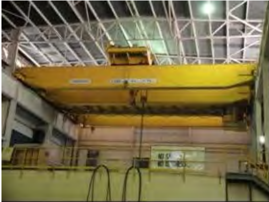
Photo 3.4-1 Overhead Crane Full View
