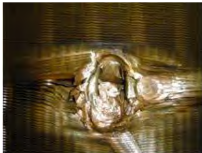
Photo 3.1-7 Damage of air cooler fin
