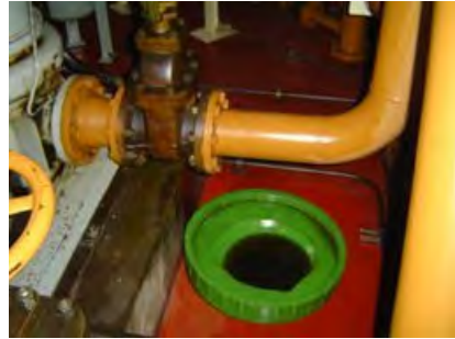
Photo 3.1-10 Oil-leaking from oil circulating pump
