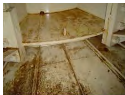
Photo 3.1-12 Oil-gathering underneath Oil Flow control valve
