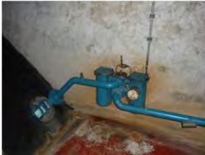
Photo 3.2-8 Filter for Shaft Seal Supply Water
