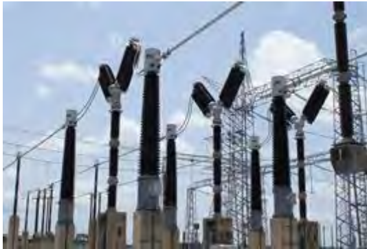
Photo 3.3-4 Old 330kV circuit breaker (BBC ELF 362 nc 2a 1983)
