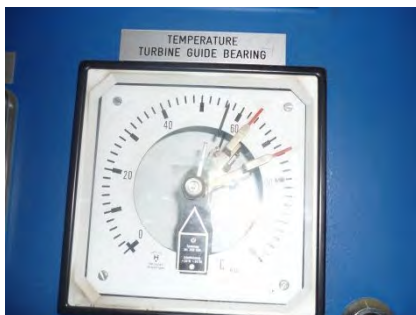
Photo-33 Turbine Guide Bearing Temperature Meter
