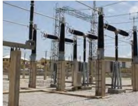
Photo 3.3-5 New 330kV circuit breaker (Areva GL315 2010)
