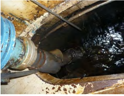
Photo-26 Water level in shaft seal
