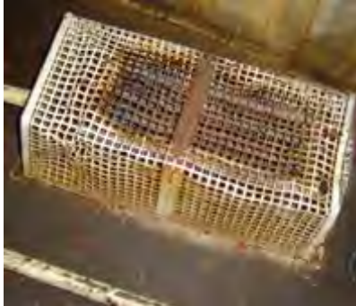
Photo 3.1-13 Deformation of space heater covers were detected
