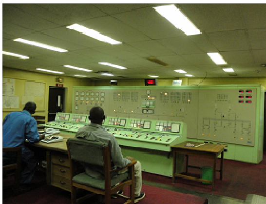
Jebba Hydroelectric Power Station Control Room
