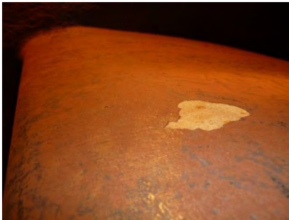
Photo-4 Paint on Stay Vane
