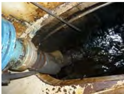
Photo 3.2-4 Water level in shaft seal
