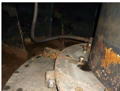
Photo-24 Shaft Seal
