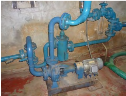
Photo-36 Water supply pump
