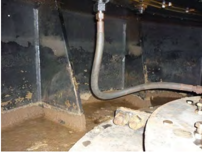
Photo-27 Shaft Seal
