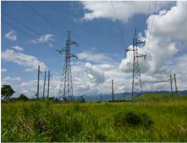
Transmission lines for Gusap (#602) and Erap (#601)
