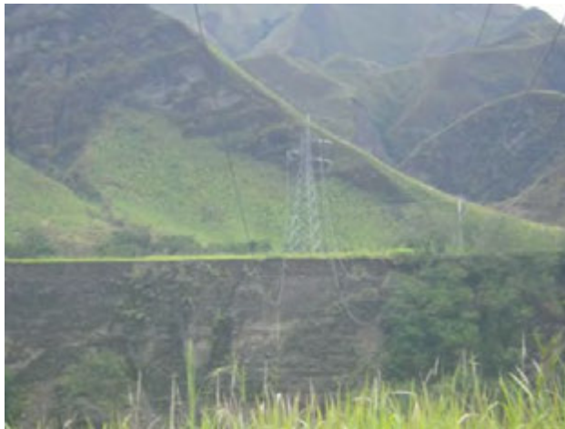
Transmission Line Crossing over the Leron River (2/2)
