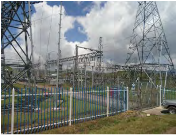
Ramu 1 Switchyard Overview
