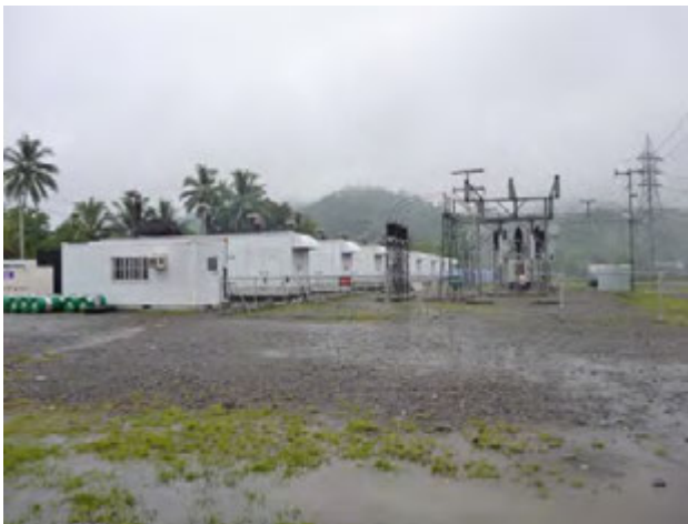
8 x 1.8 MW Diesel Engine Generators
