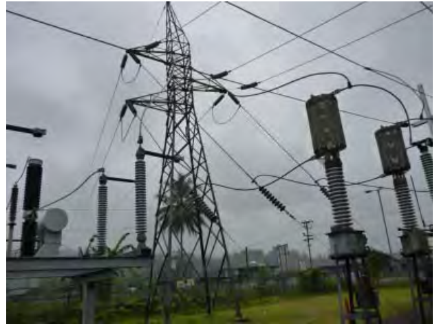
132 kV Tower for Erap
