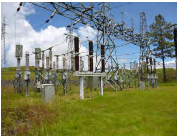
132 kV Circuit Breaker
