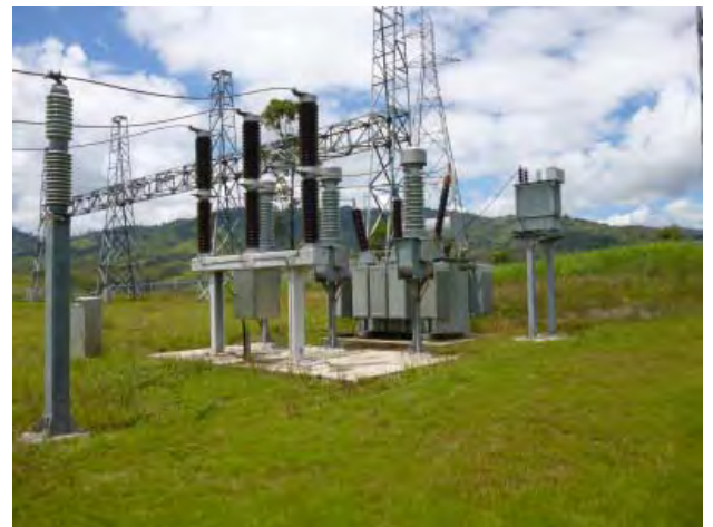
132/22 kV Distribution Transformer
