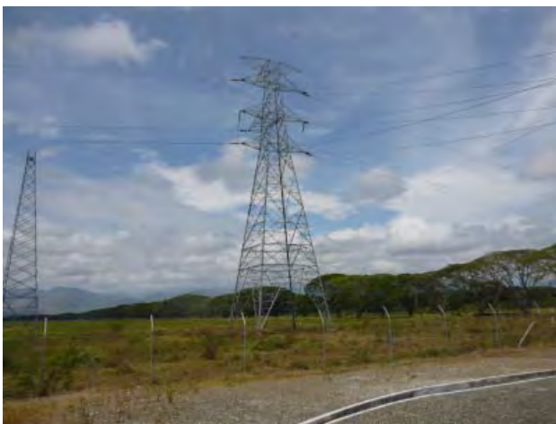
Double Circuit Tower
