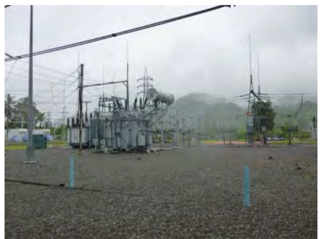
No.1 Main Transformer 132/66 kV, 15/20 MVA
