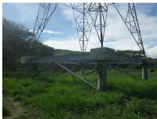
Bent Pile Foundation
