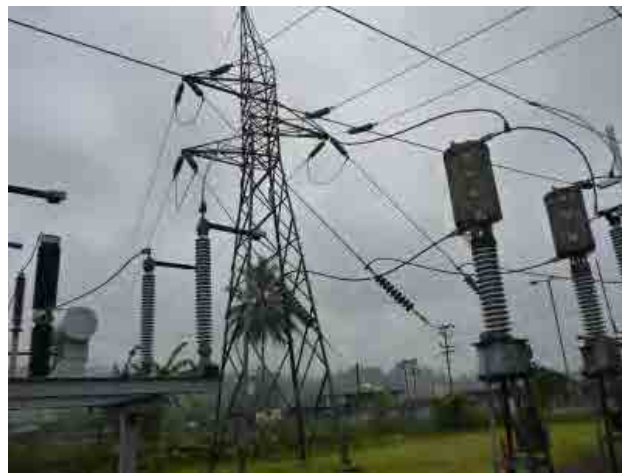
132 kV Tower for Erap
