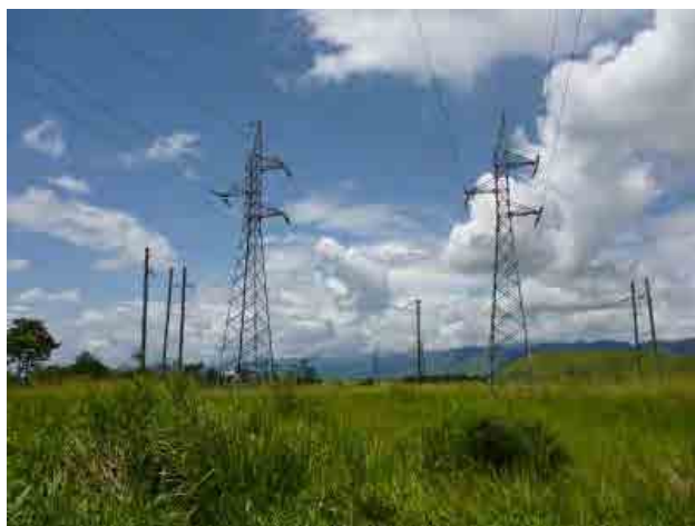
Transmission lines for Gusap (#602) and Erap (#601)
