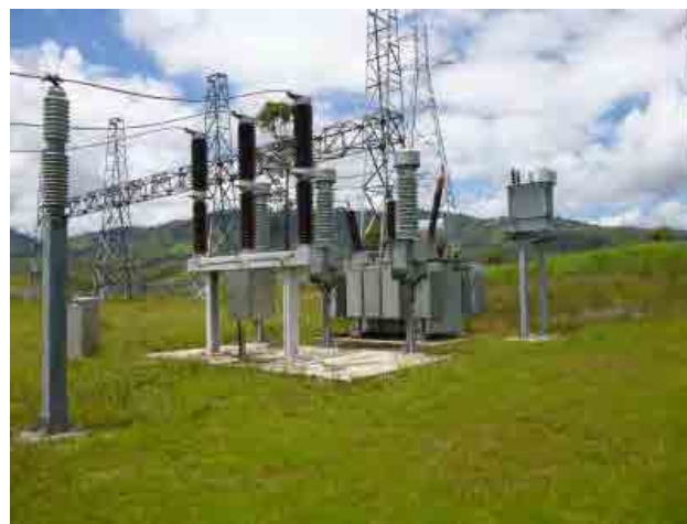
132/22 kV Distribution Transformer
