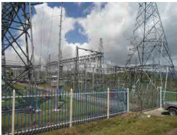
Ramu 1 Switchyard Overview
