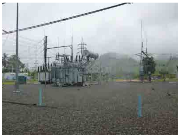
No.1 Main Transformer 132/66 kV, 15/20 MVA
