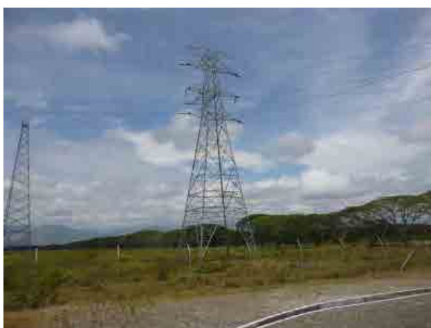
Double Circuit Tower
