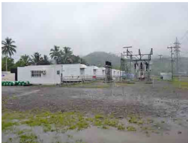
8 x 1.8 MW Diesel Engine Generators
