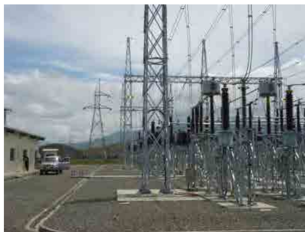
Transmission Line to Hidden Valley SS
