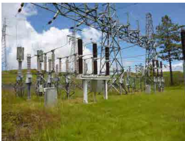
132 kV Circuit Breaker
