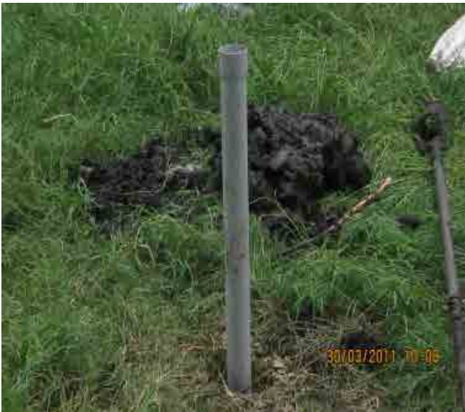
Stand Pipe for Piezometer Measurement
