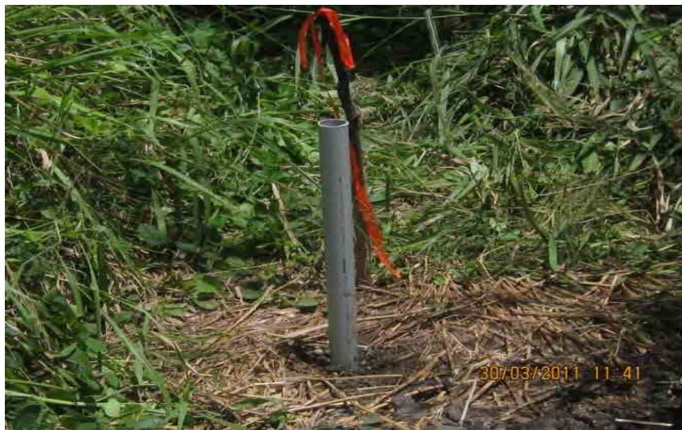
Stand Pipe for Piezometer Measurement
