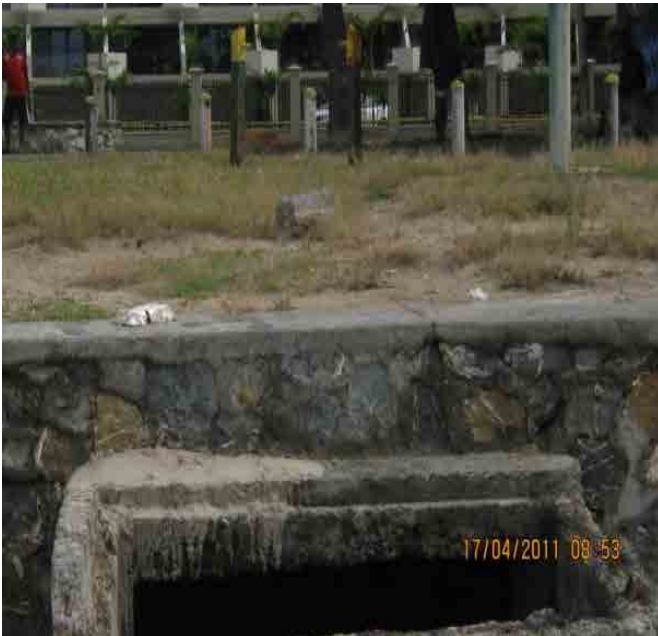
Sewerage outlet to the sea
