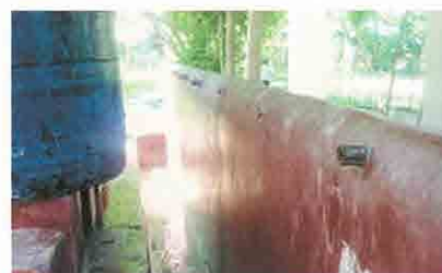
Even Taps of the Plant were stolen away
