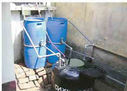
Simple Water Treatment Plant
