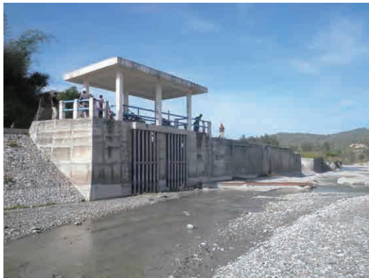
Intake portion of present intake facility (2 intake gates have not been operated due to severe siltation at intake gate portion, sediment trap basin and irrigation canal.)
