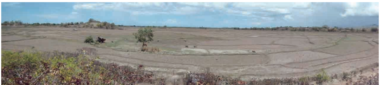
Irrigation area of the Buluto irrigation project (Main canal is constructed front of the photograph with flow direction of from left to right)
