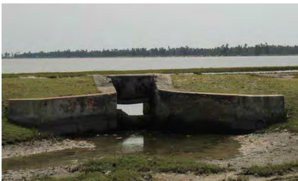
Figure 7: Damaged Salt water exclusion bund at Mandaithivu, Velanai DS
